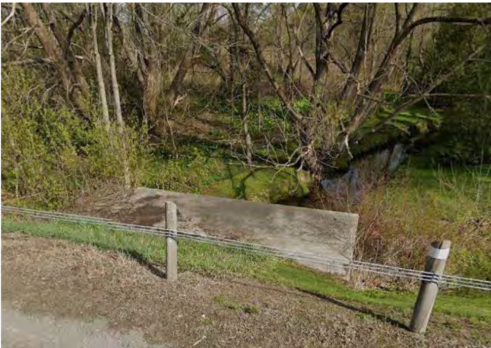
Image 16 Creek has been disturbed by construction of the concrete culvert carrying creek under Fourteenth Street West
