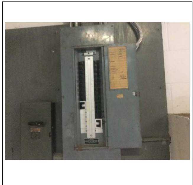
Photo 4: Old electrical panel and main switch.
