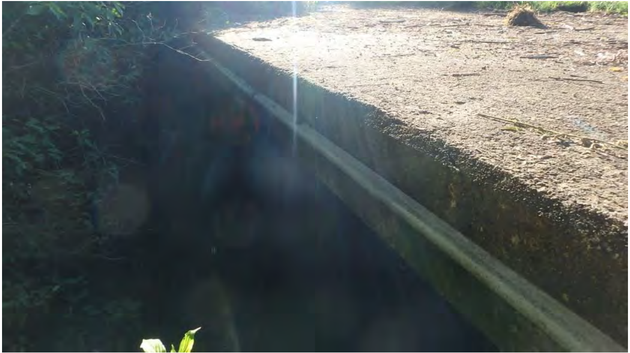
Figure 11 Utility Attached at Inlet
