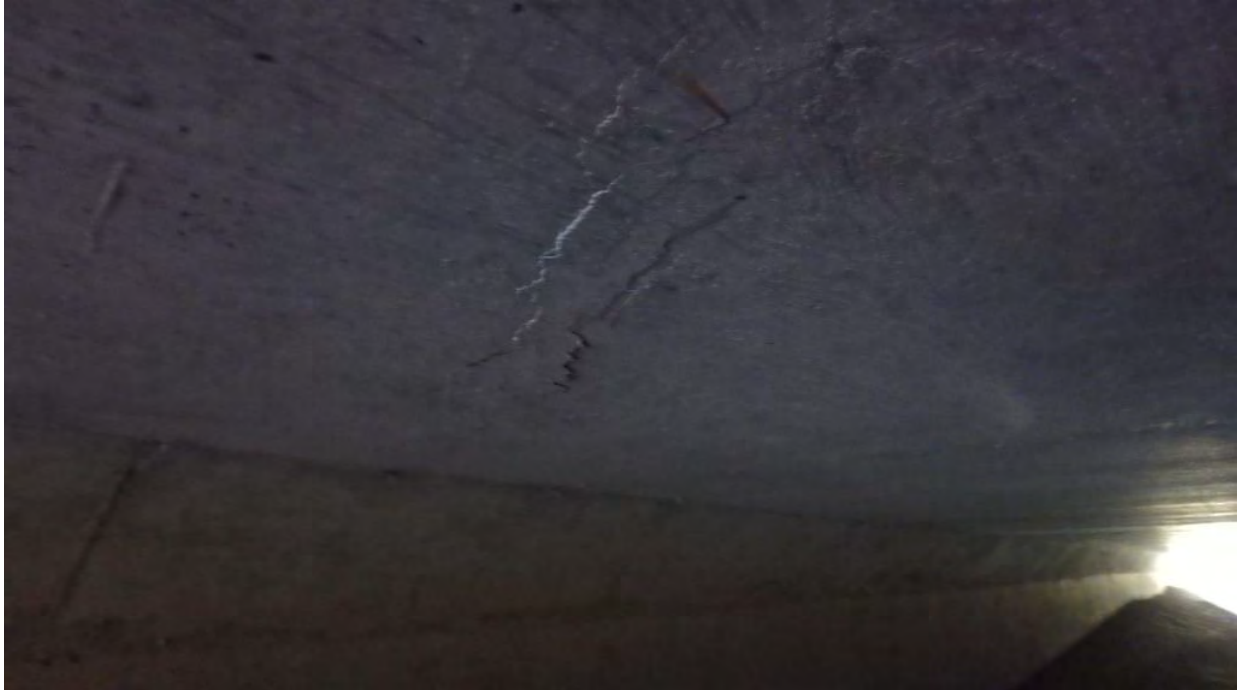
Figure 8 Narrow Crack in Soffit
