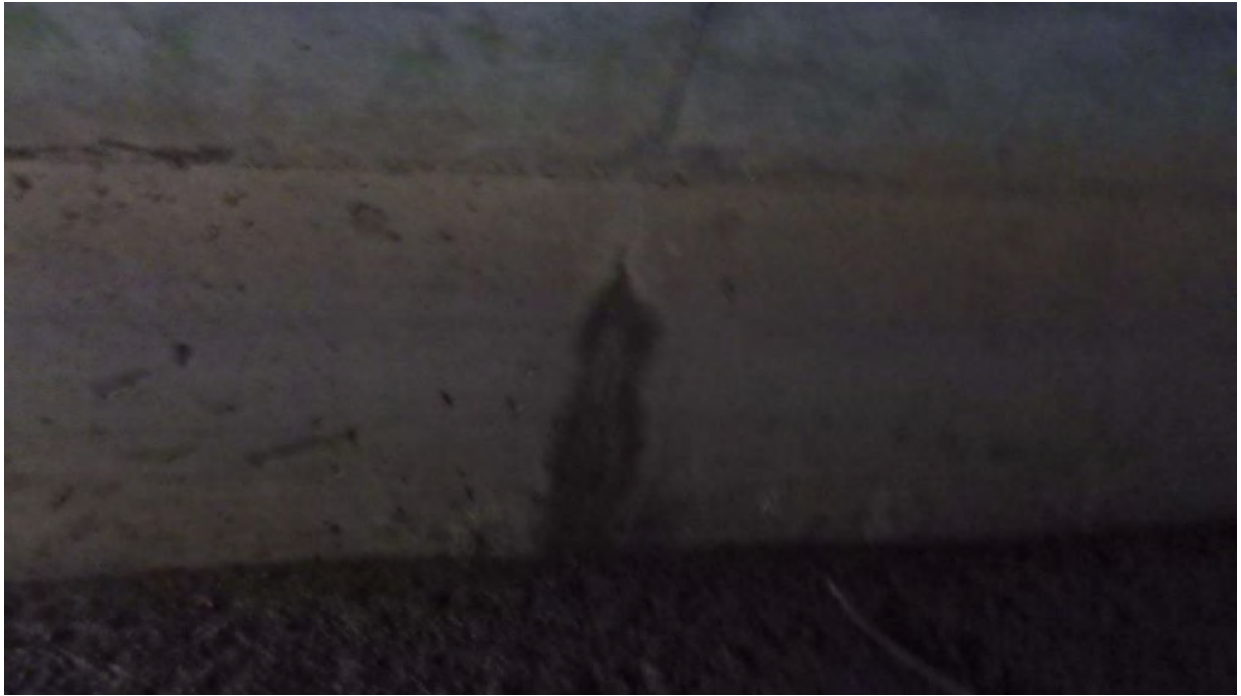
Figure 9 Narrow Vertical Crack in West Wall
