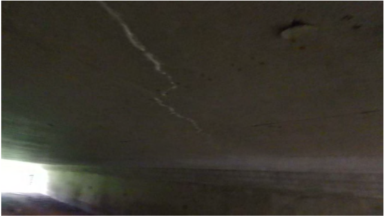
Figure 9 Transverse Soffit Crack
