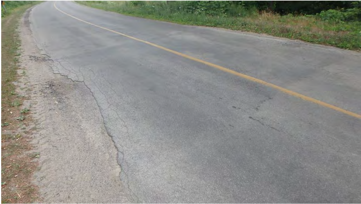
Figure 10 Settlement and Edge Deterioration in Wearing Surface at Culvert
