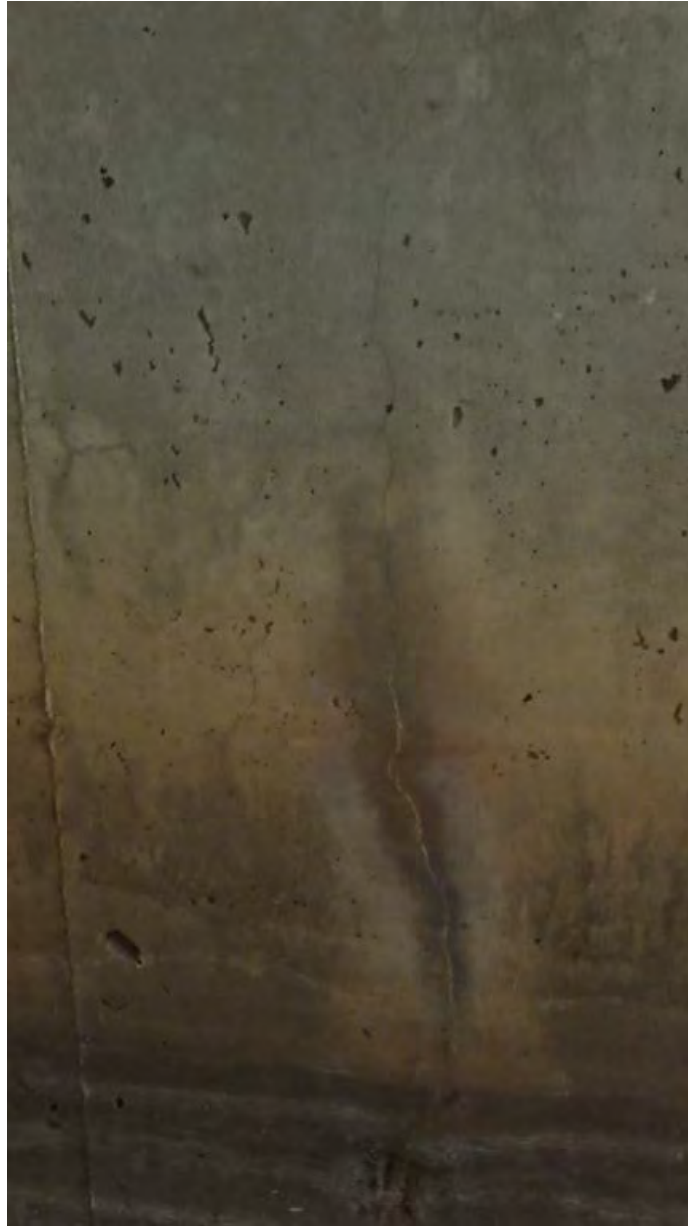
Figure 9 Typical Crack on Wall with Staining
