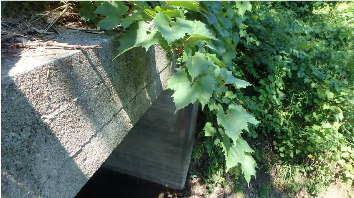
Figure 8 Minor Deterioration on South Fascia
