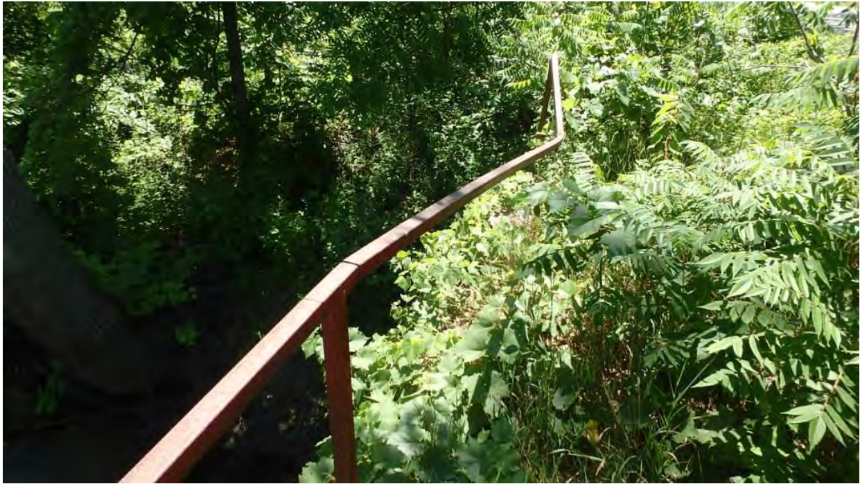
Figure 11 Damaged Handrail on South Culvert Top
