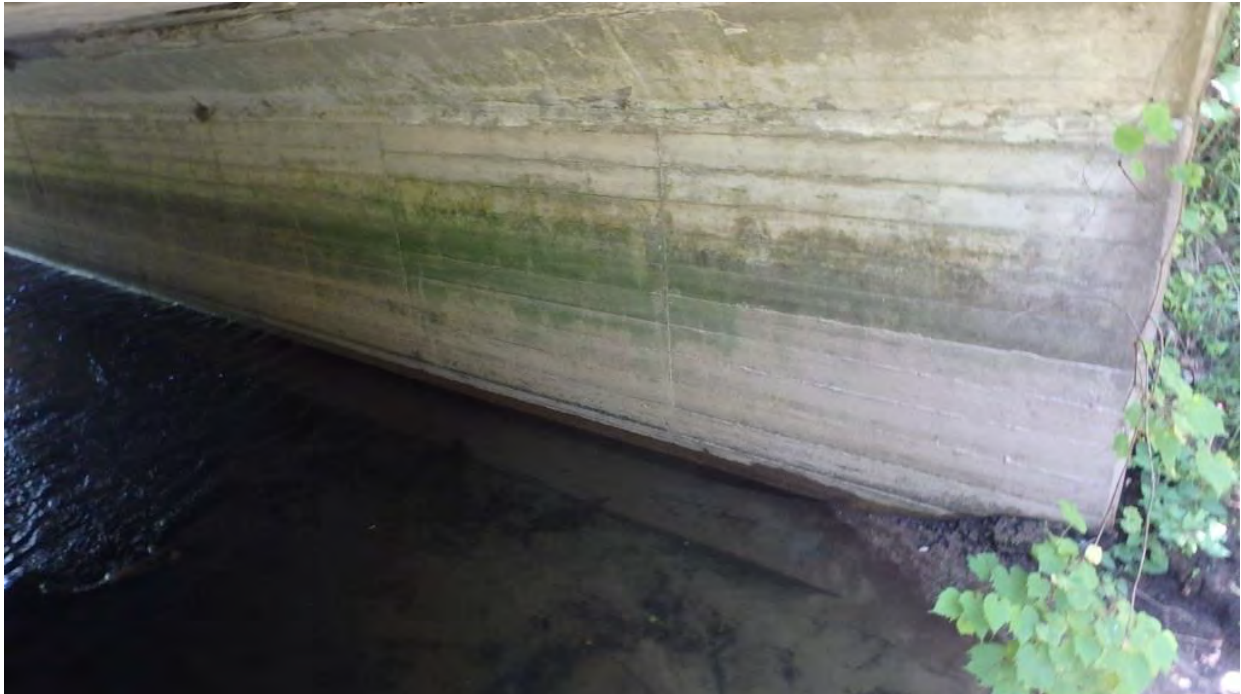
Figure 10 Staining on Culvert Walls
