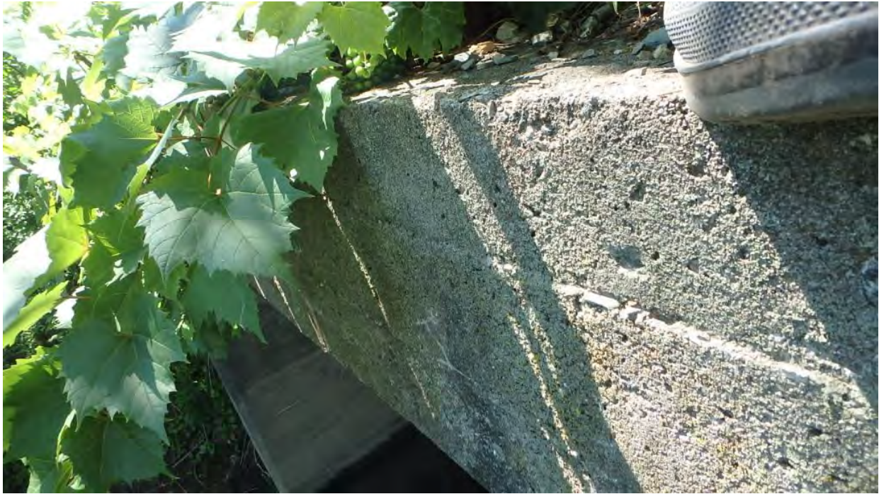
Figure 9 Scaling on Fascia
