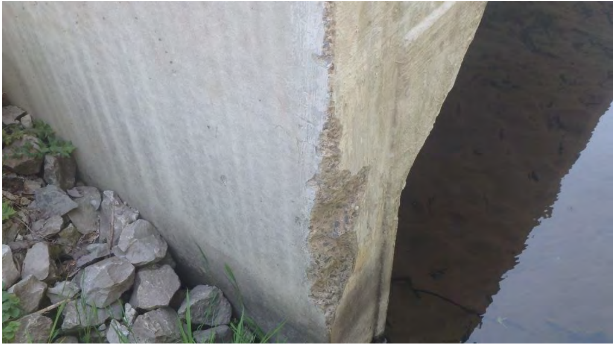
Figure 9 Minor Impact Damage in Southeast Quadrant
