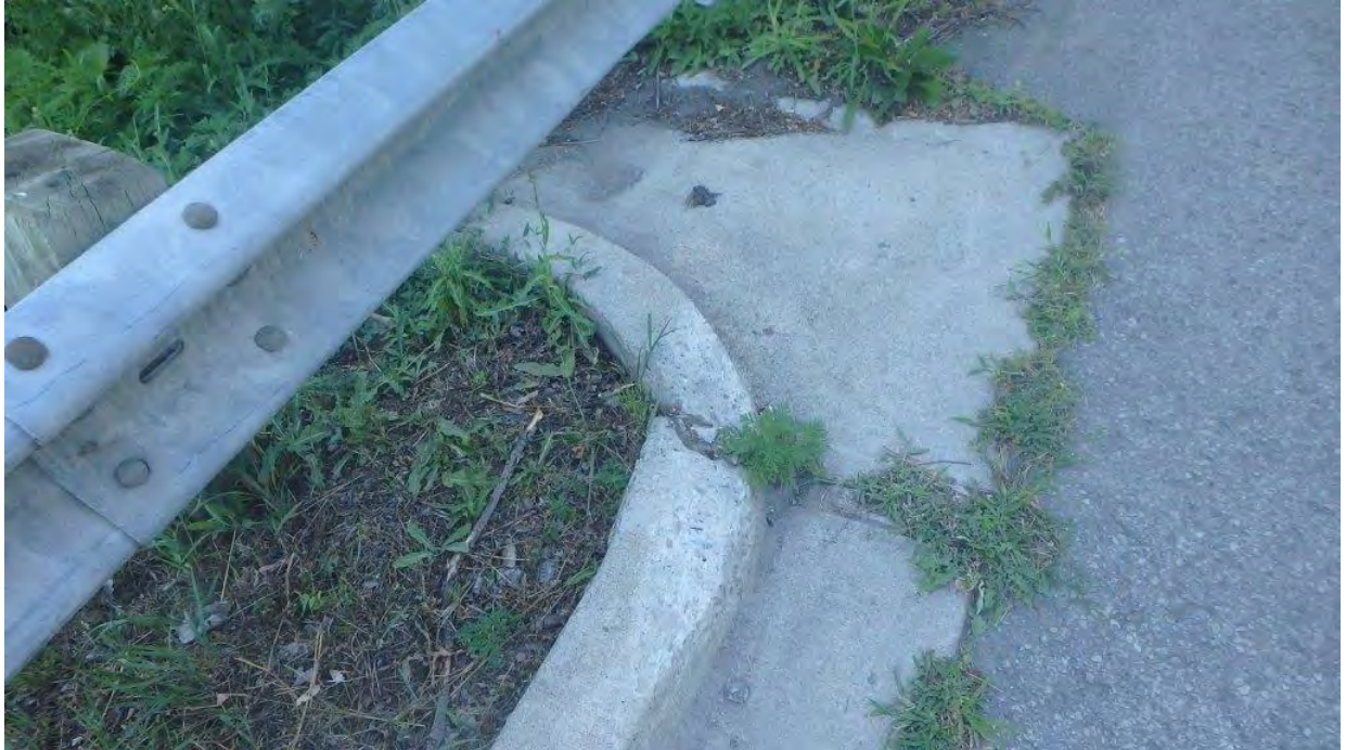
Figure 12 Minor Impact Damage at Curb
