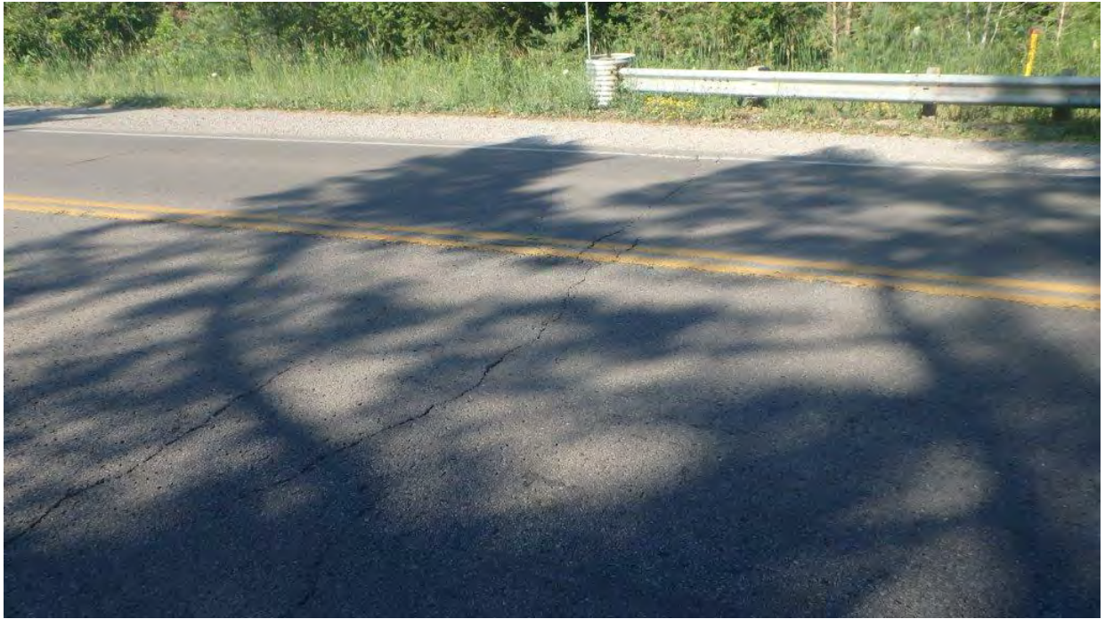
Figure 11 Transverse Cracks in Wearing Surface Approaches
