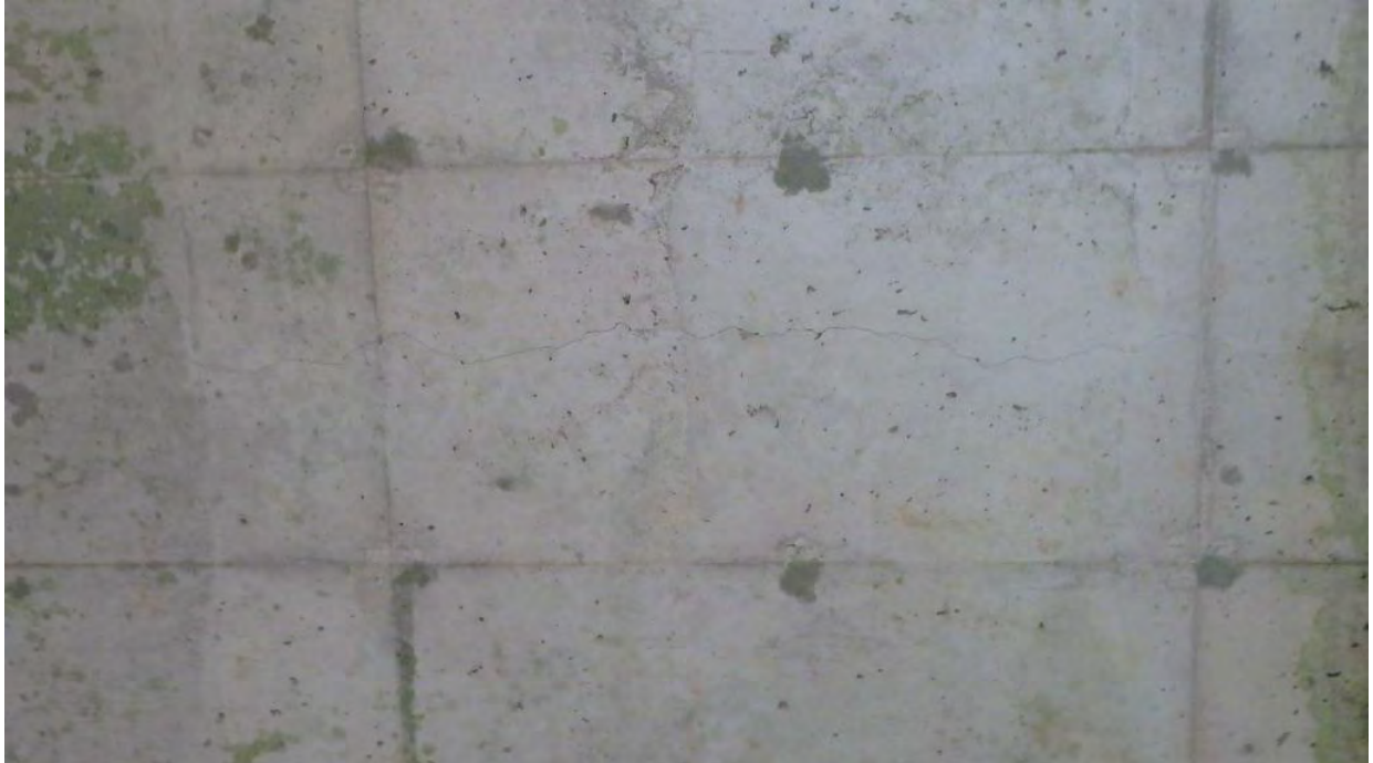
Figure 10 Vertical Hairline Crack in South Wall
