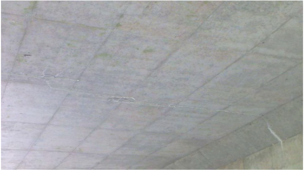
Figure 12 Crack in Soffit with Leakage & Chlorides
