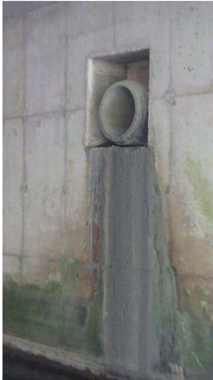
Figure 11 Staining & Minor Deterioration at Drains
