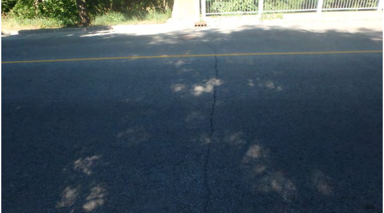
Figure 15 Transverse Crack in Wearing Surface
