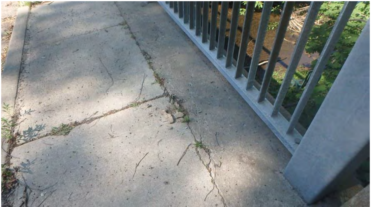
Figure 13 Crack & Spall in Sidewalks
