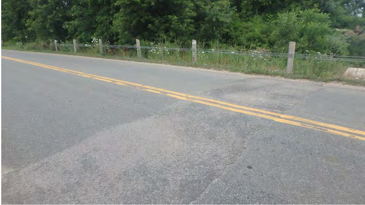
Figure 15 Large Patch at West Approach with apparent Settlement
