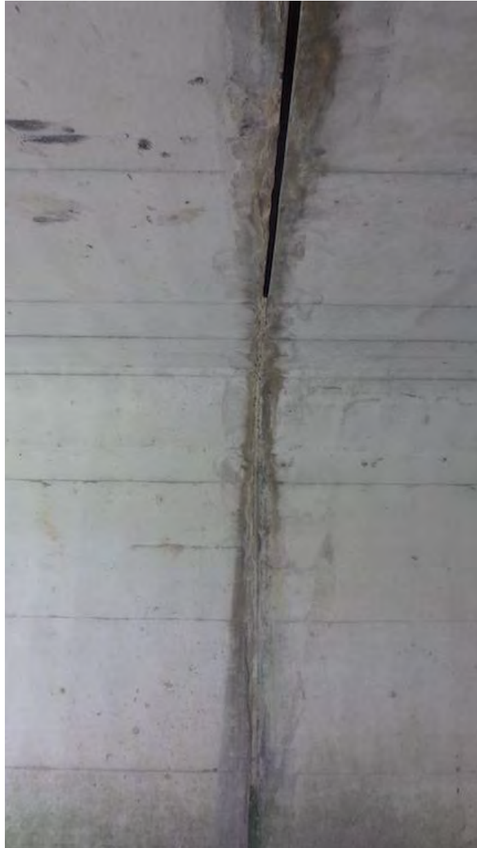
Figure 13 Cracking and Deterioration of Parging at Joint with Chlorides
