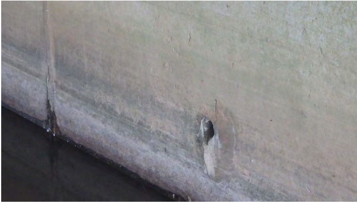
Figure 11 Drains with Staining
