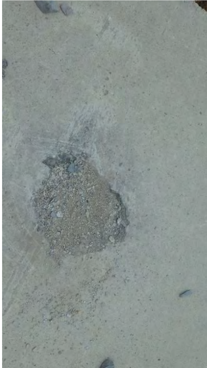
Figure 14 Failing of Parging at Lifting Hooks
