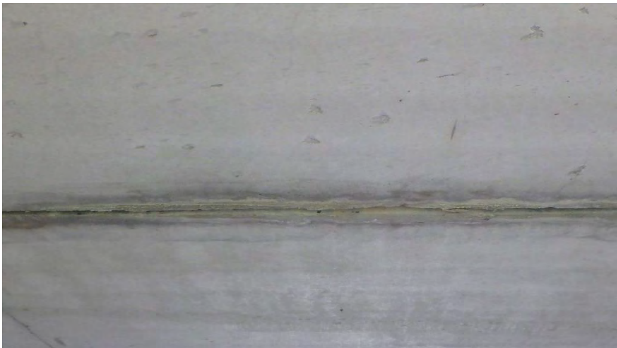
Figure 12 Leakage and Chlorides at Joints
