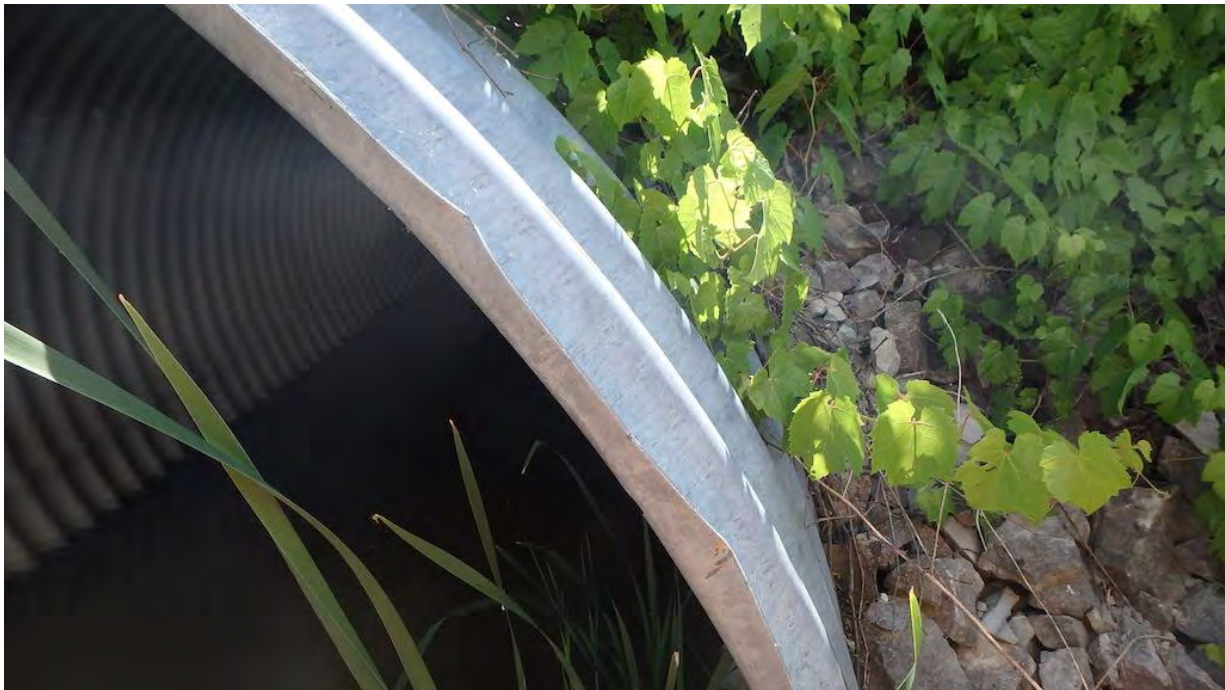
Figure 10 Minor Impact Damage on Culvert
