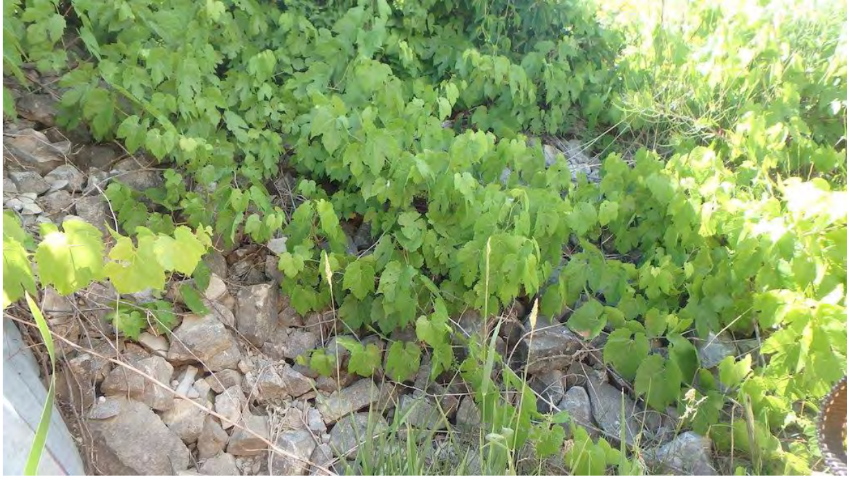
Figure 9 Minor Erosion at Northeast Quadrant
