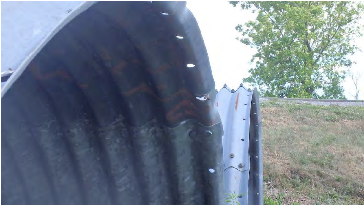
Figure 10 Minor Installation Damage
