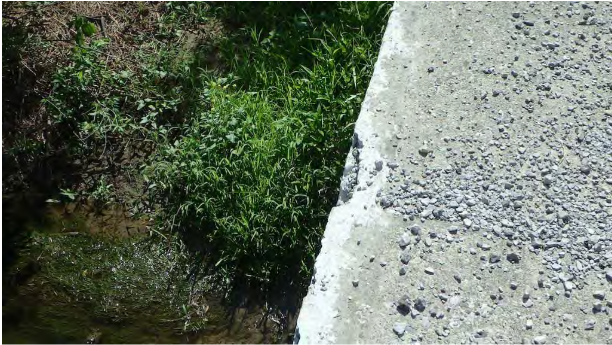
Figure 11 Small Spall at South Culvert
