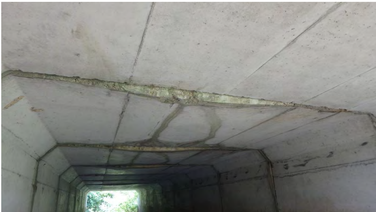
Figure 12 Typical Leakage at Precast Joints
