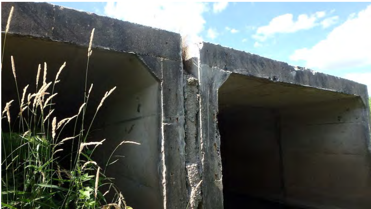
Figure 10 Separation of Parging Between Culvert at South Side
