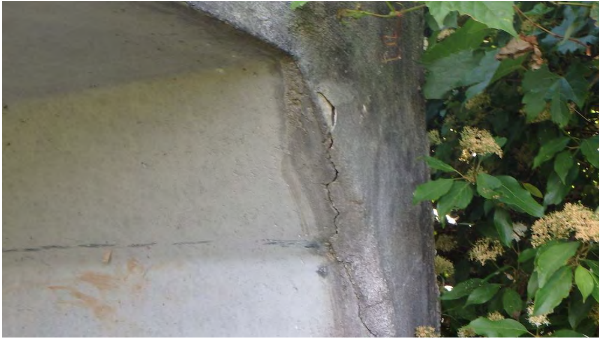
Figure 9 Light Delamination at Northwest Quadrant
