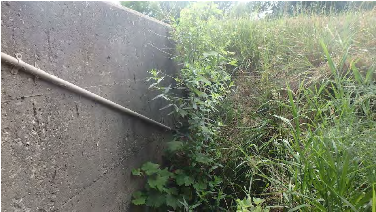
Figure 10 Minor Erosion at Northeast Quadrant
