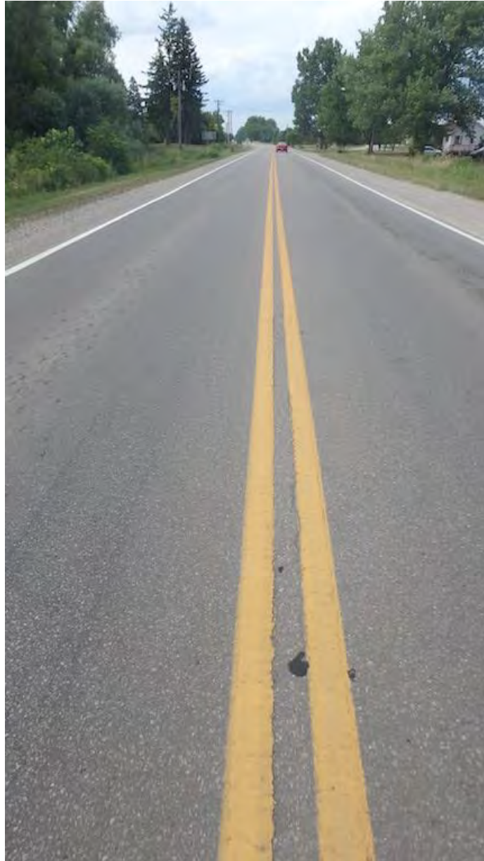
Figure 9 Small Longitudinal Cracks in Wearing Surface at Centreline
