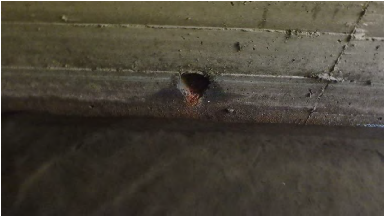
Figure 7 Staining and Scaling at Drains
