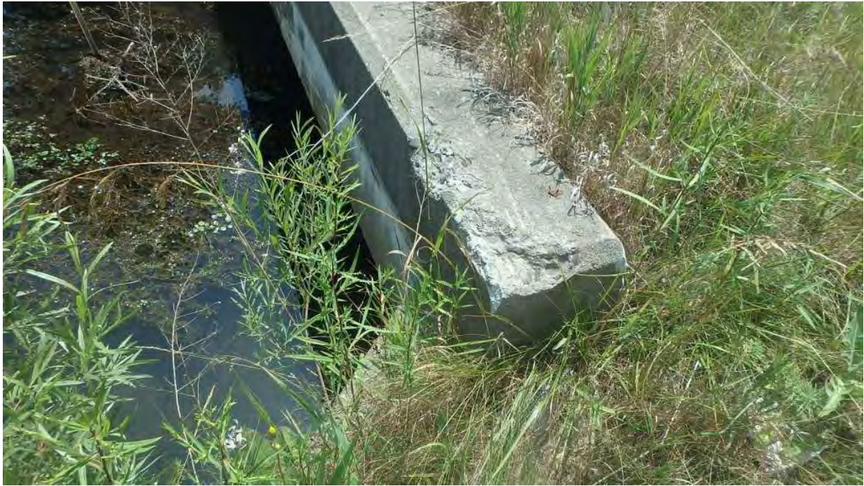
Figure 11 Impact Damage at NE Quadrant
