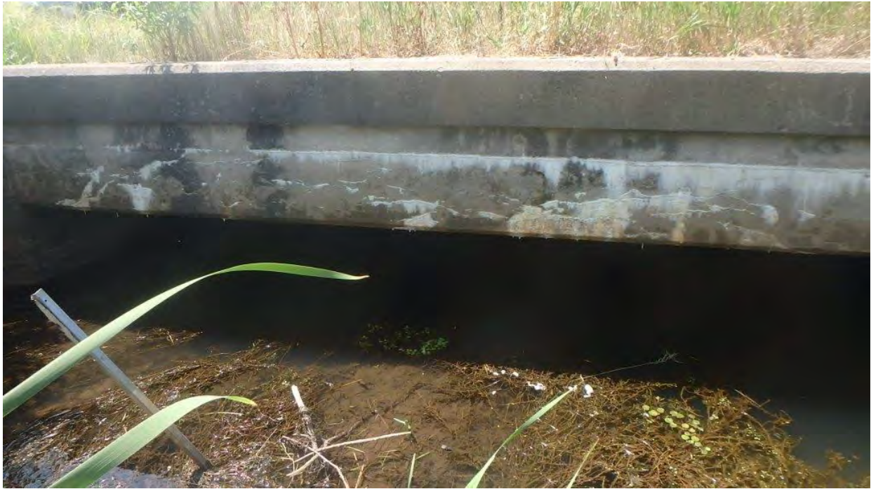
Figure 9 Hairline Cracking and Efflorescence at East
