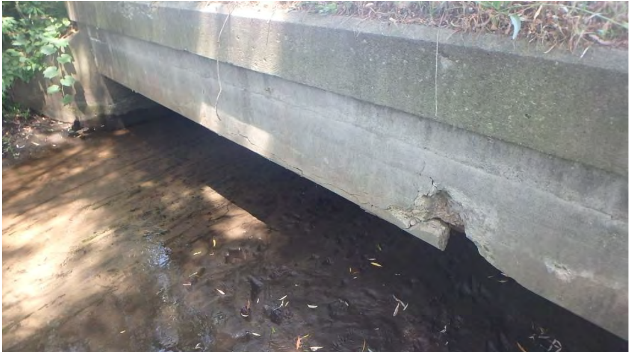
Figure 10 Crack and Spall at West End
