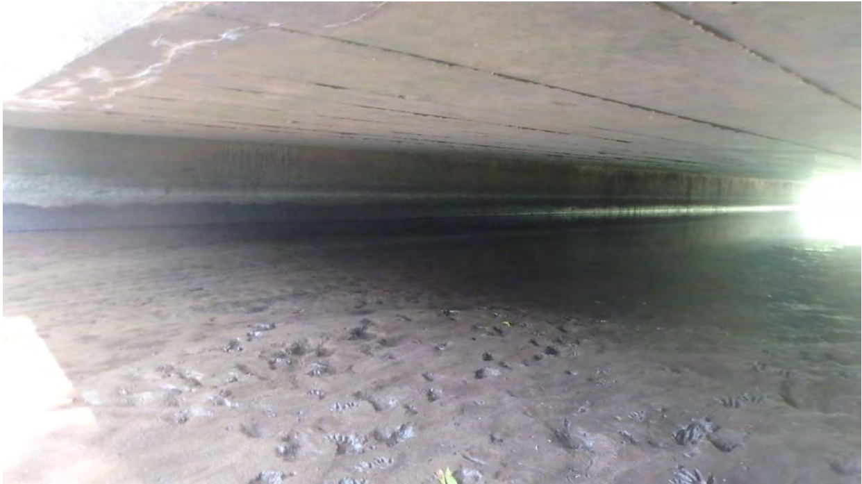
Figure 8 Soffit and North End, Note Amount of Fill
