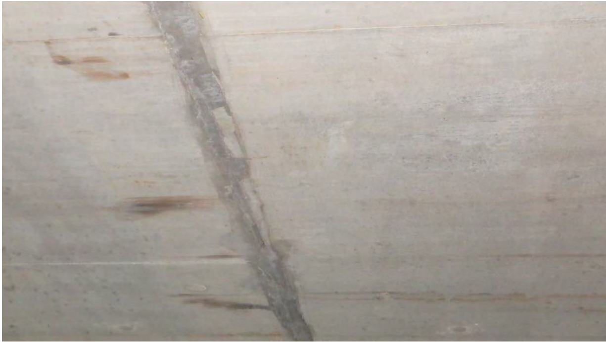
Figure 9 Parging Failing at Interior Joints
