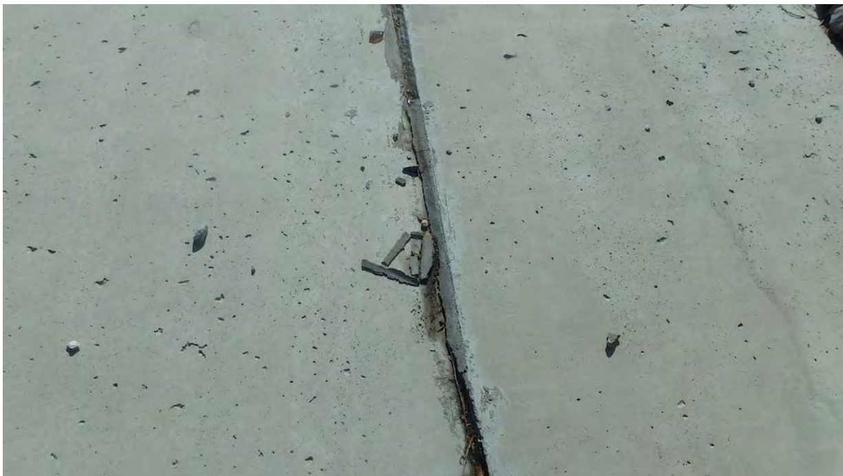
Figure 10 Parging Failing at Joints
