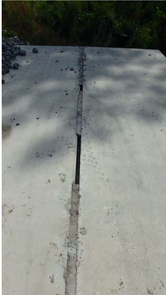
Figure 9 Wide Box Joint at South, Parging Failing and Leaking
