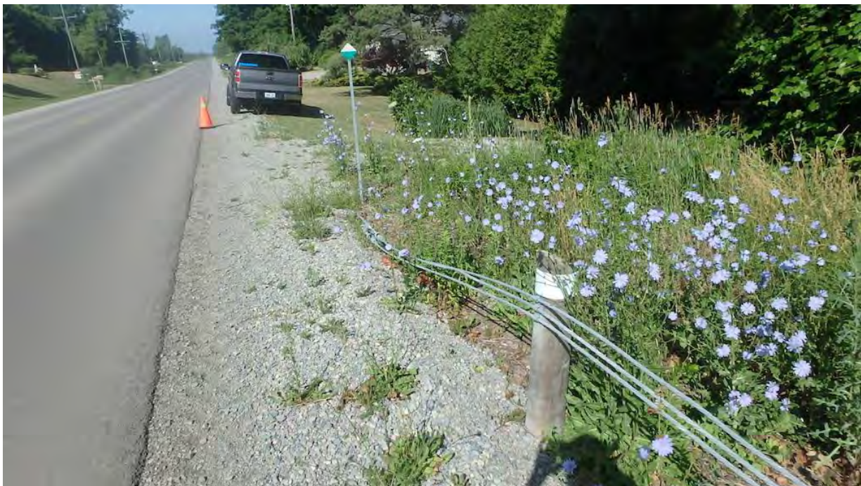
Figure 11 Loose Guiderail Cables
