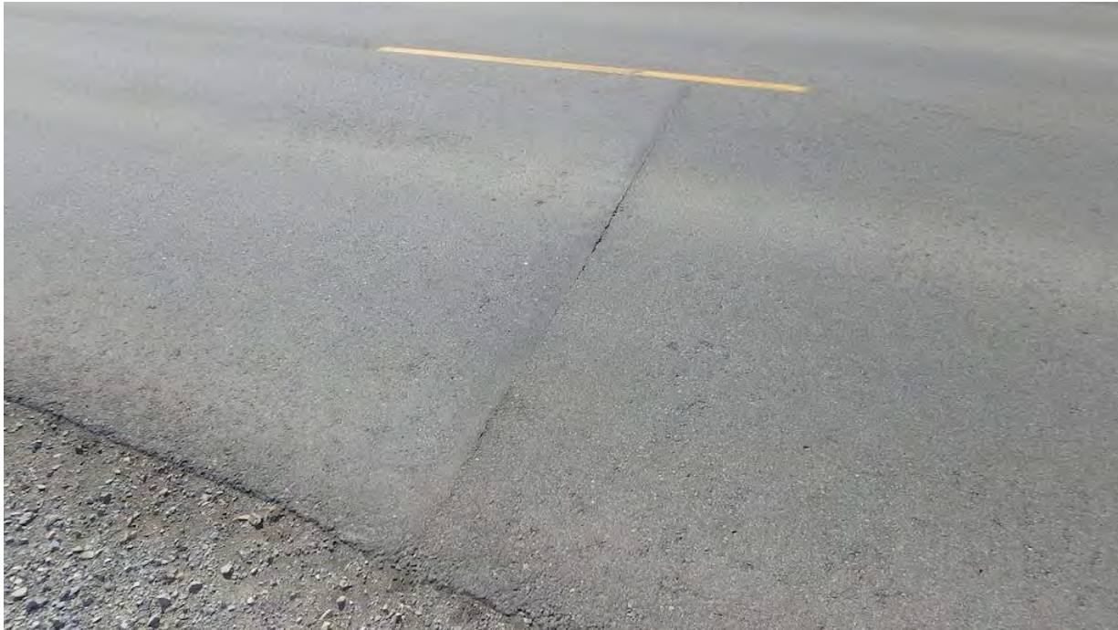
Figure 10 Transverse Crack in Wearing Surface
