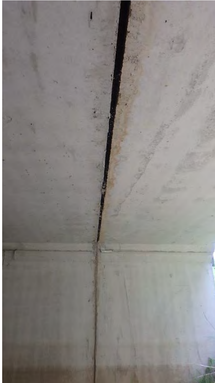
Figure 8 South Box Joint Leaking
