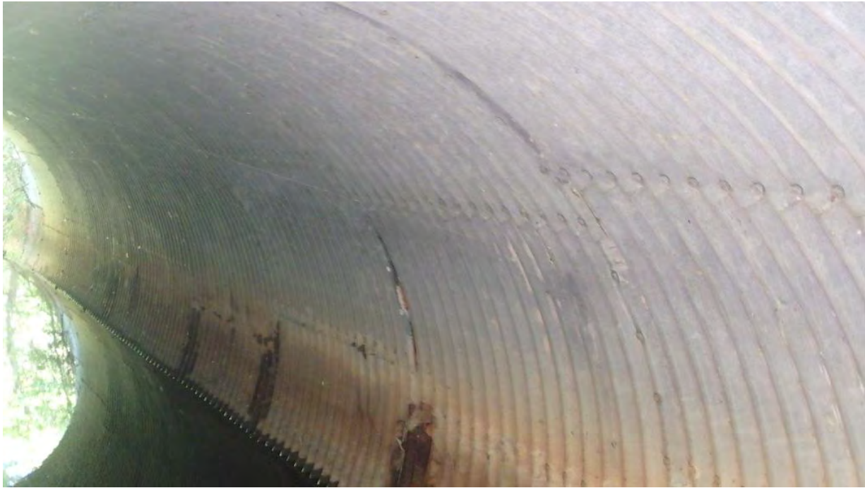
Figure 9 Areas of Corrosion and Leakage in Barrel
