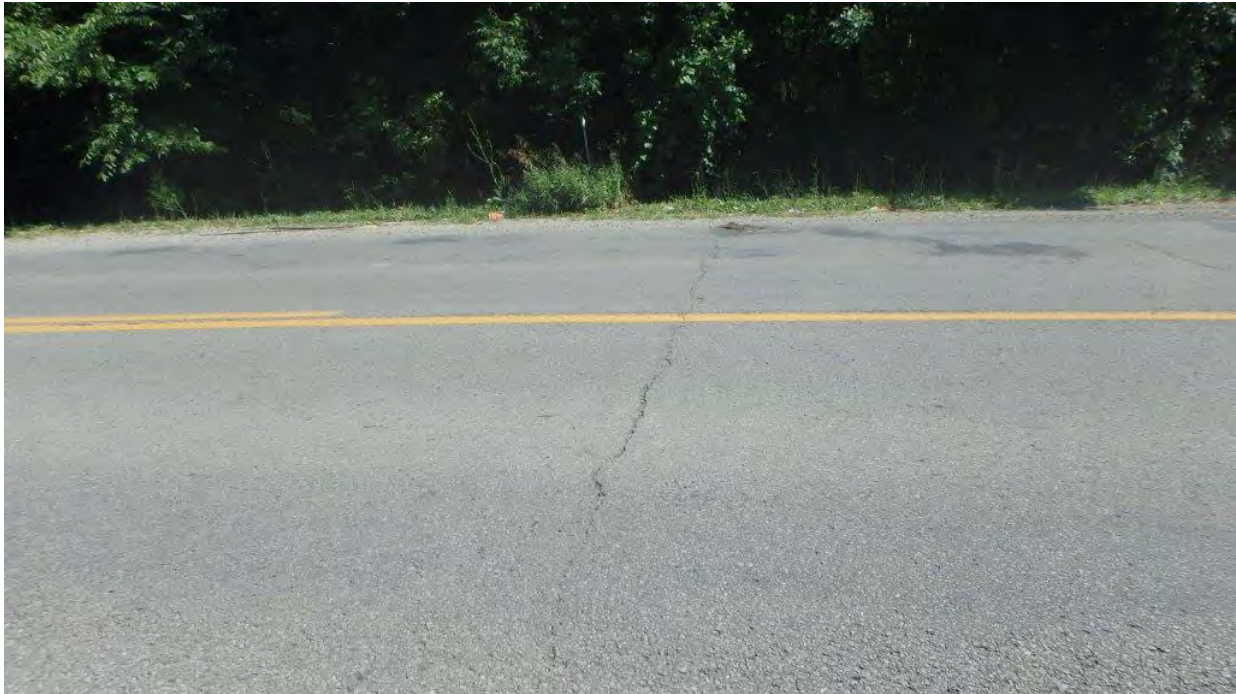
Figure 11 Transverse Crack in Wearing Surface
