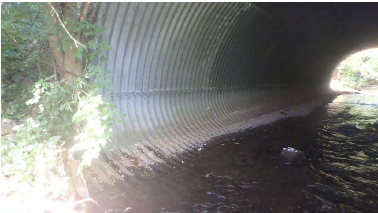
Figure 10 Typical Water level Staining & Corrosion
