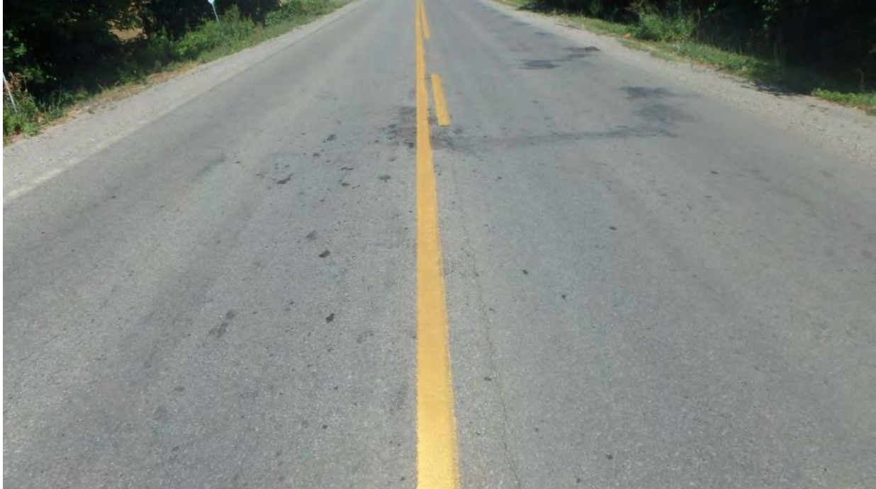
Figure 12 Longitudinal Crack in Wearing Surface
