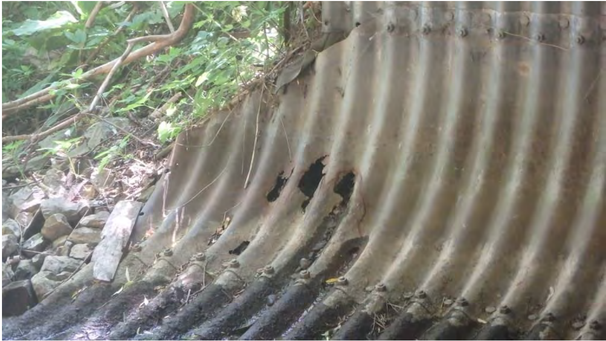
Figure 9 Deteriorated Holes in Culvert at South
