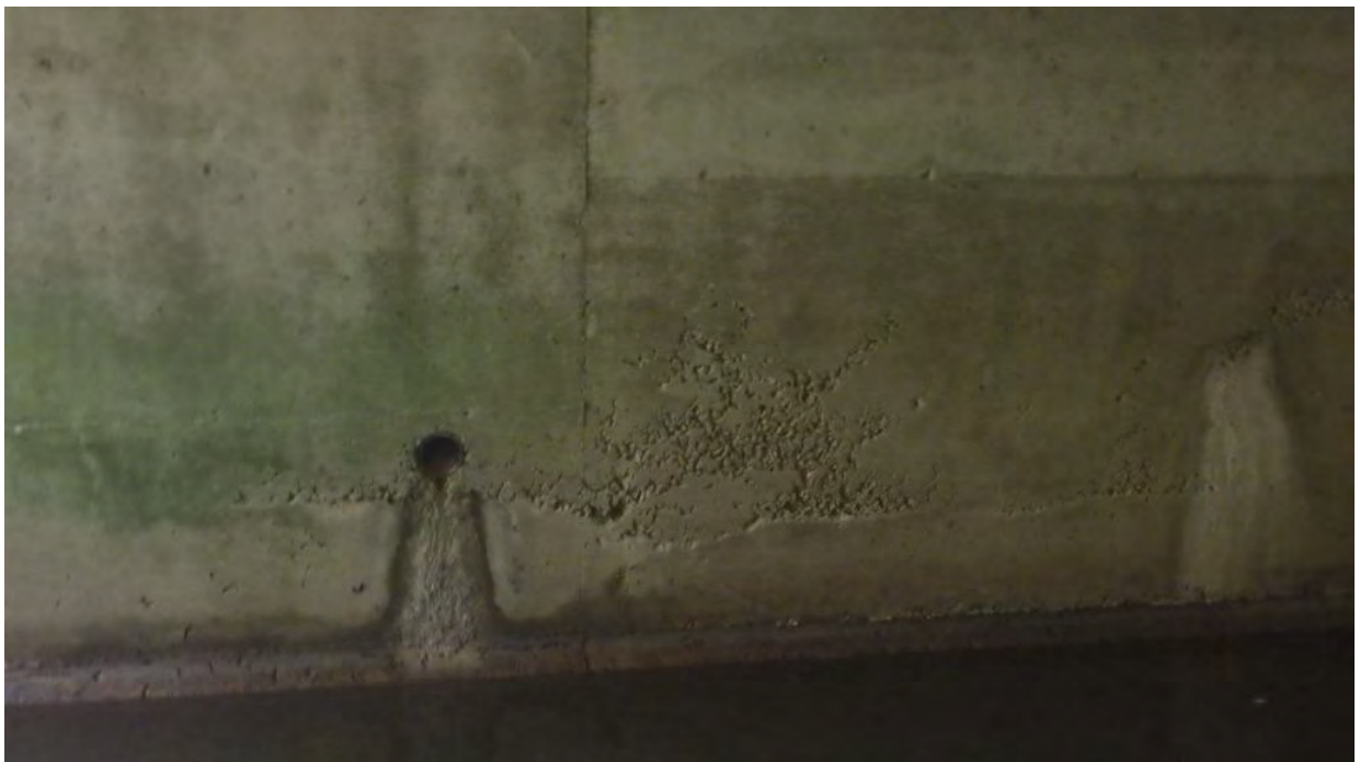
Figure 12 Leakage & Staining at Drains
