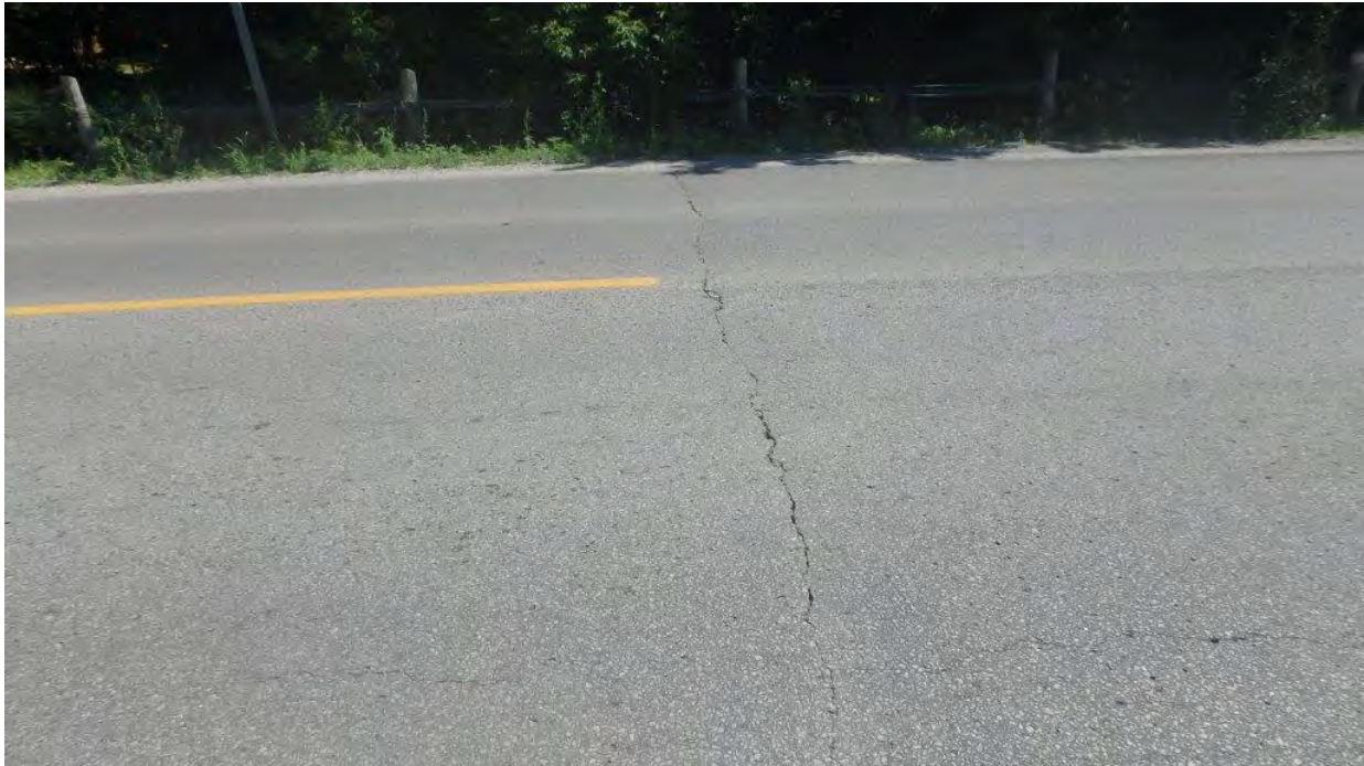
Figure 15 Typical Transverse Crack in Wearing Surface
