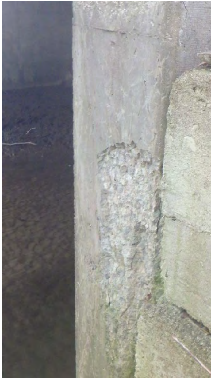
Figure 13 Large Spall at Northwest Quadrant
