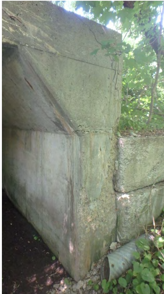
Figure 14 Severe Spalling & Delamination with Leakage & Chlorides at Southeast Quadrant
