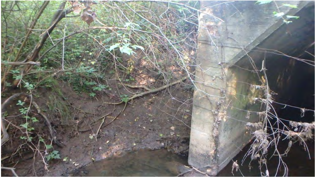
Figure 9 Minor Erosion at all Quadrants
