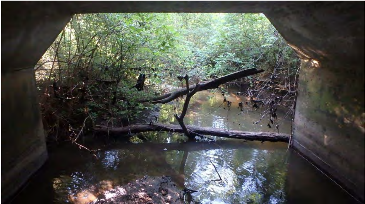
Figure 8 Debris Blockage at Inlet
