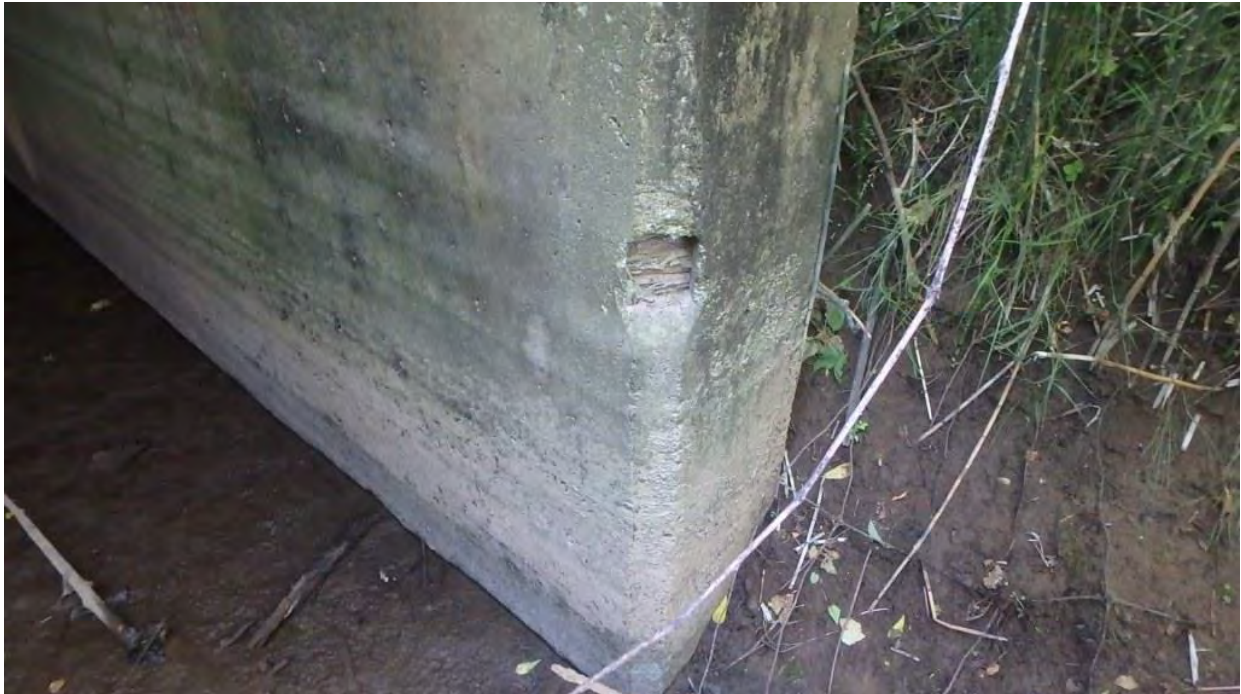
Figure 10 Wood Pop-out in Concrete at Outlet
