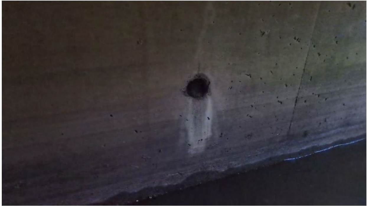
Figure 11 Staining and Hairline Crack at Drains
