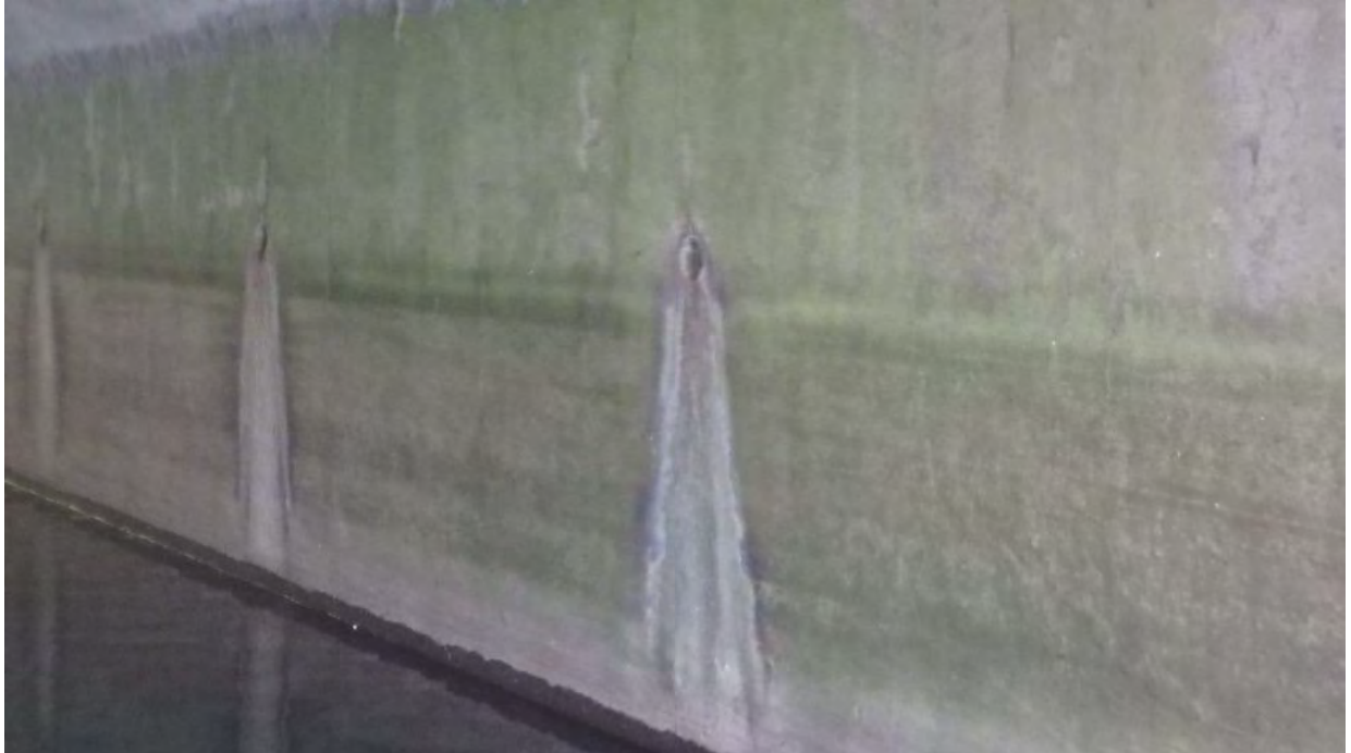
Figure 10 Staining at drains
