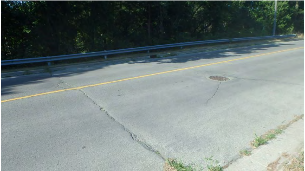
Figure 15 Transverse Cracks in Wearing Surface at Culvert Joints
