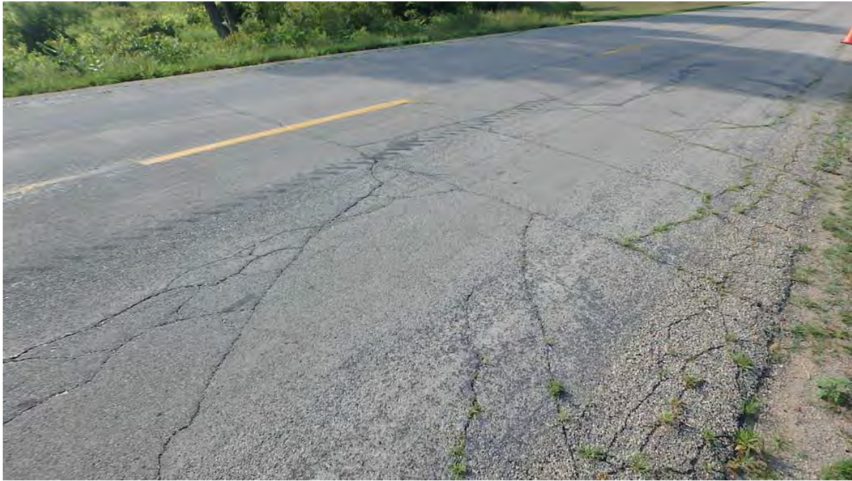
Figure 11 Cracking on Wearing Surface
