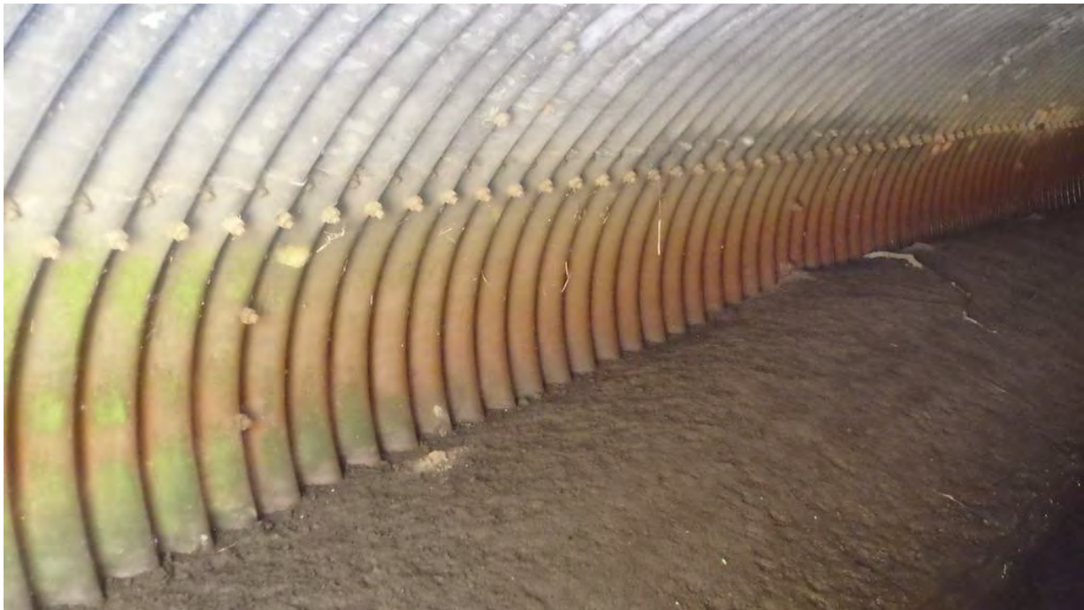
Figure 10 Corrosion at Waterline
