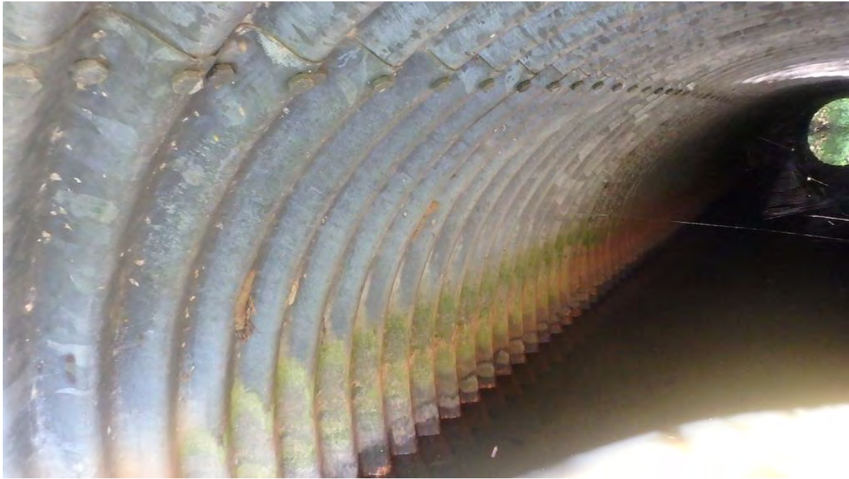
Figure 7 Corrosion at Waterline
