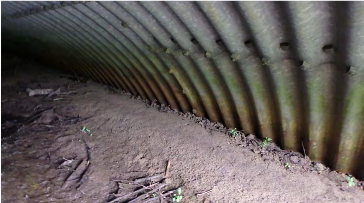
Figure 12 Corrosion, Staining at Water Line
