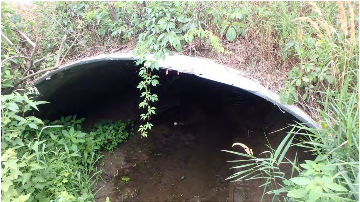
Figure 11 Damage at Top of Inlet
