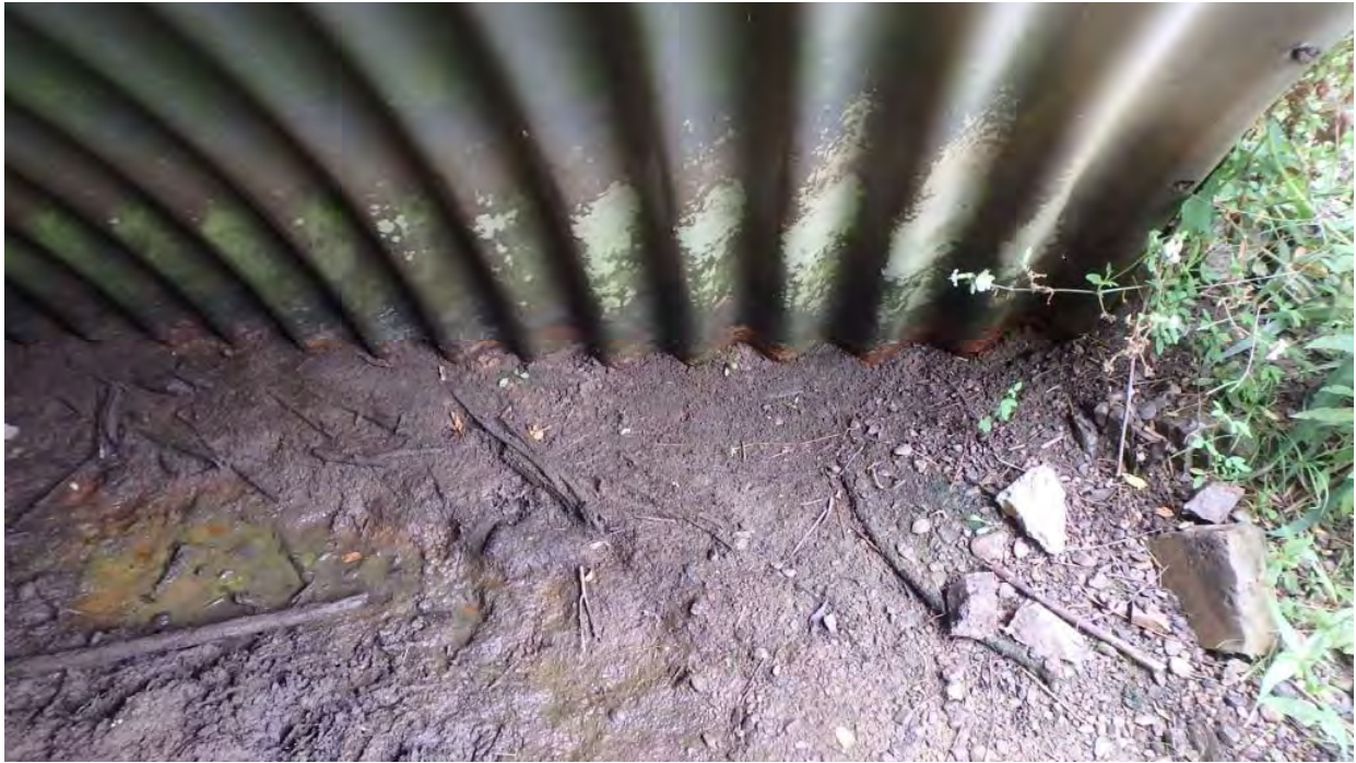
Figure 9 Corrosion at Outlet
