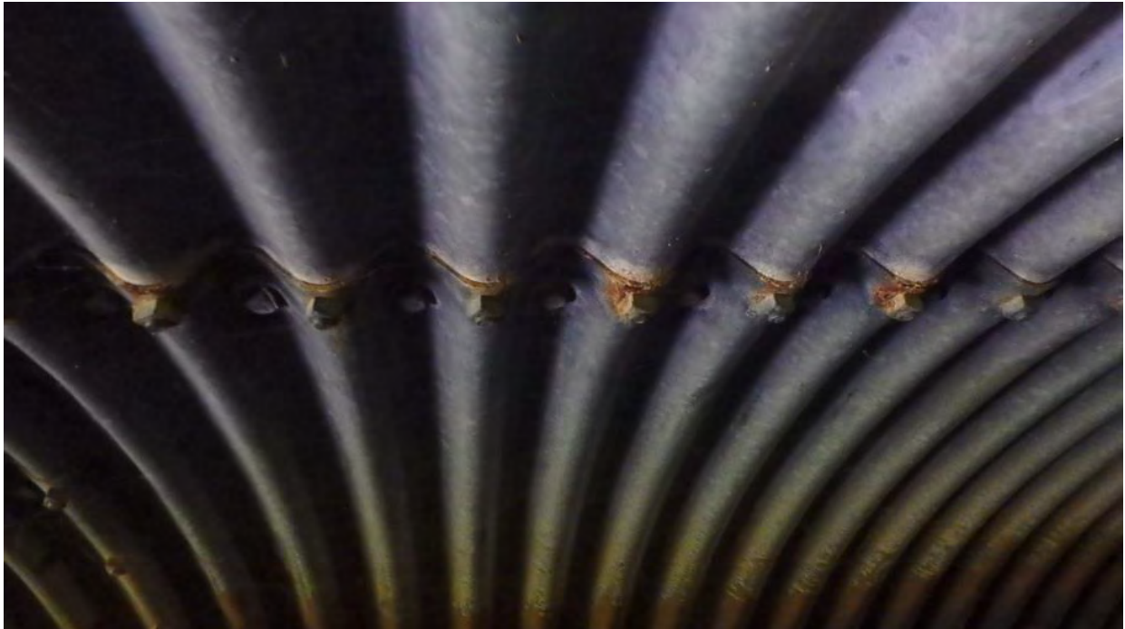
Figure 10 Corrosion of Bolts
