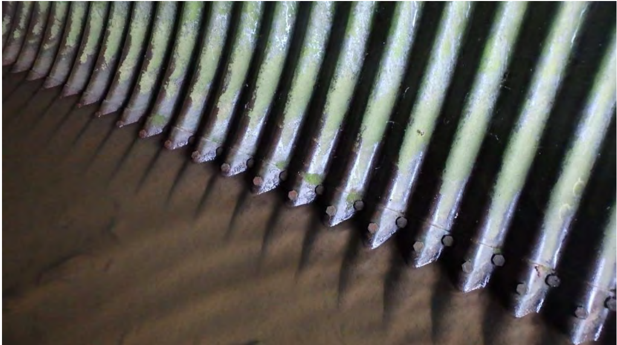
Figure 8 Corrosion and Staining at Water Line
