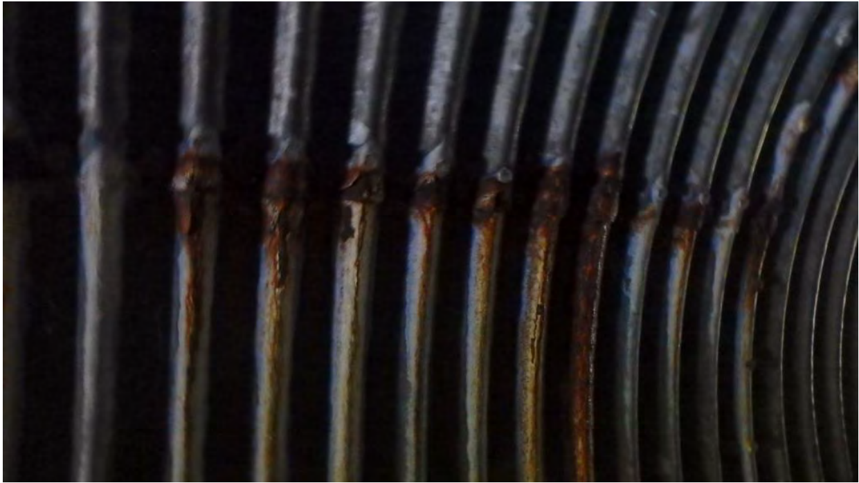
Figure 9 Corrosion at Plate Joints
