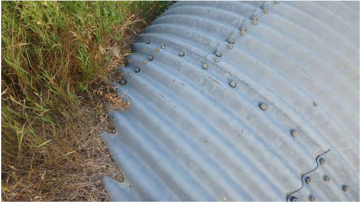
Figure 11 Minor Damage and Rusting on Culvert at Inlet
