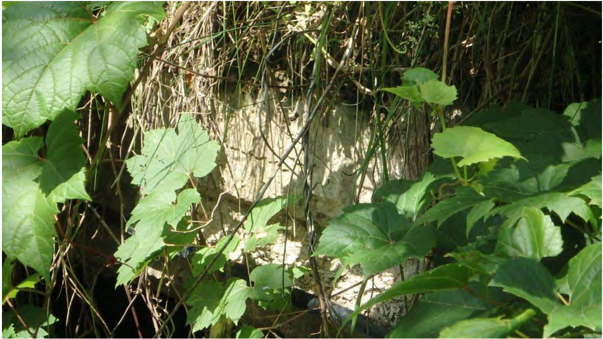
Figure 9 West Fascia Deterioration
