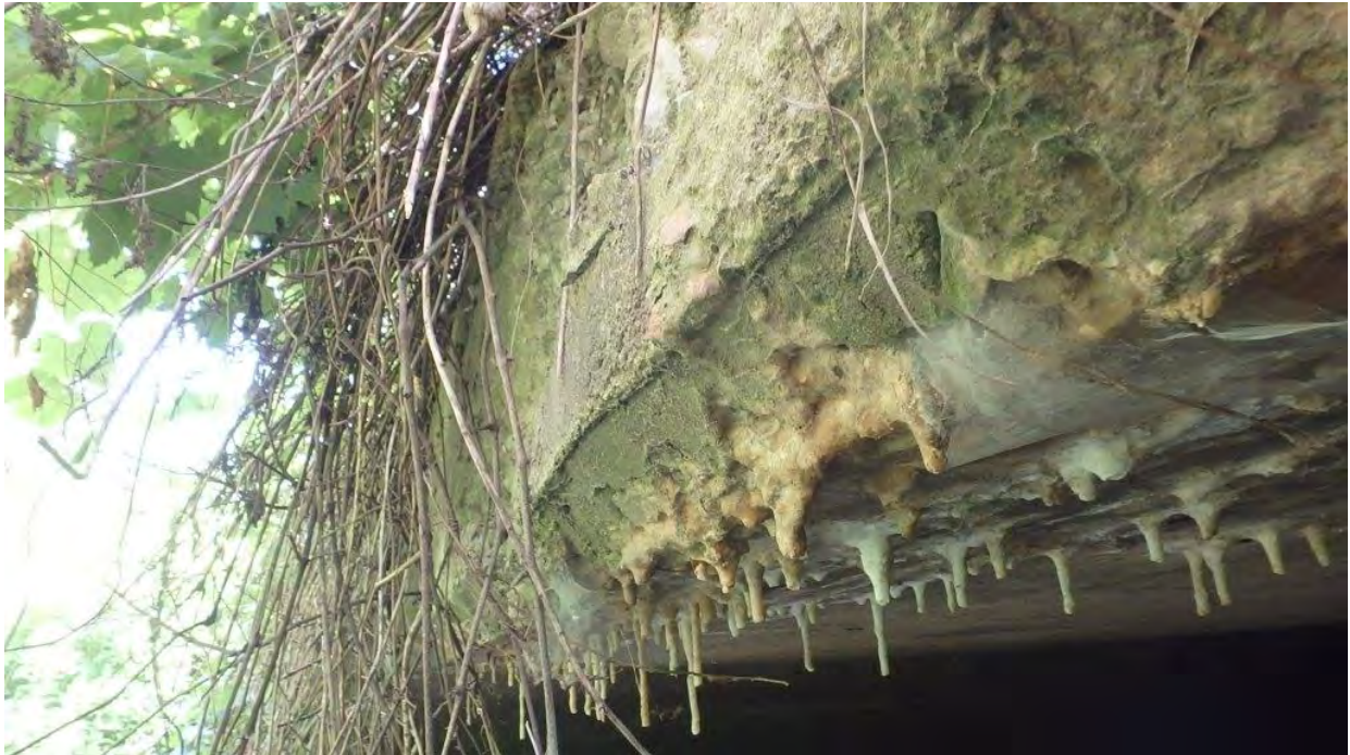
Figure 8 East Fascia Deterioration, Efflorescence & Stalactites
