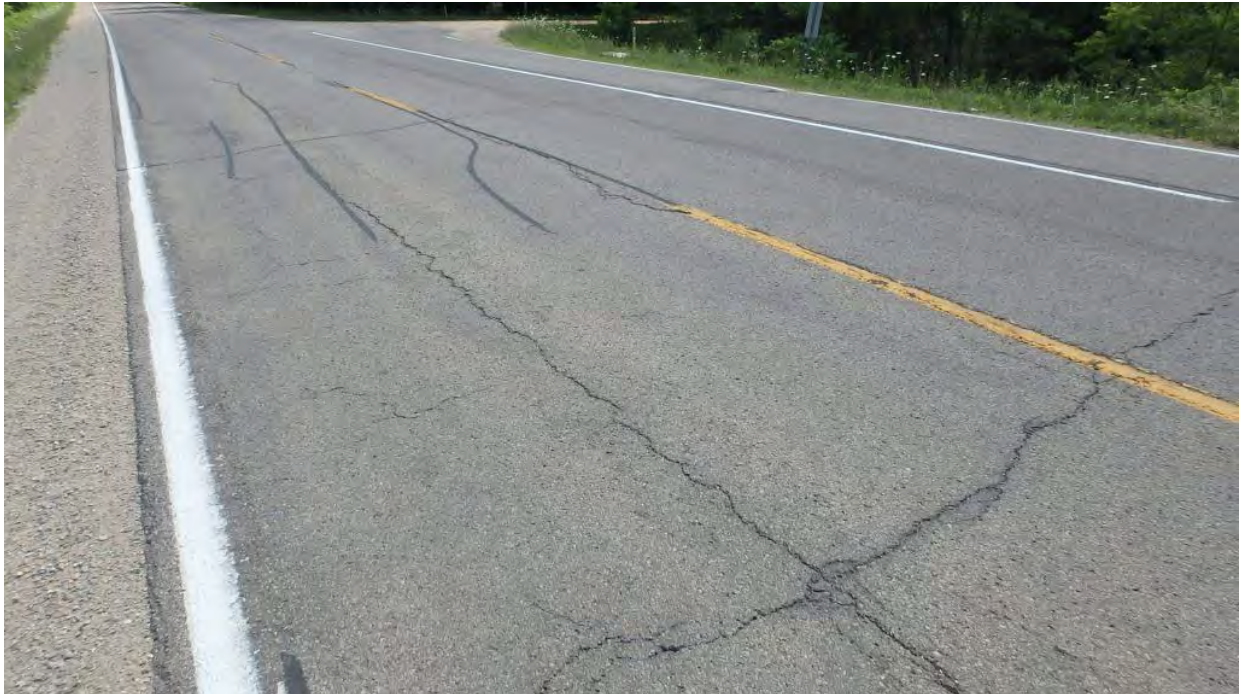
Figure 10 Cracks in Wearing Surface
