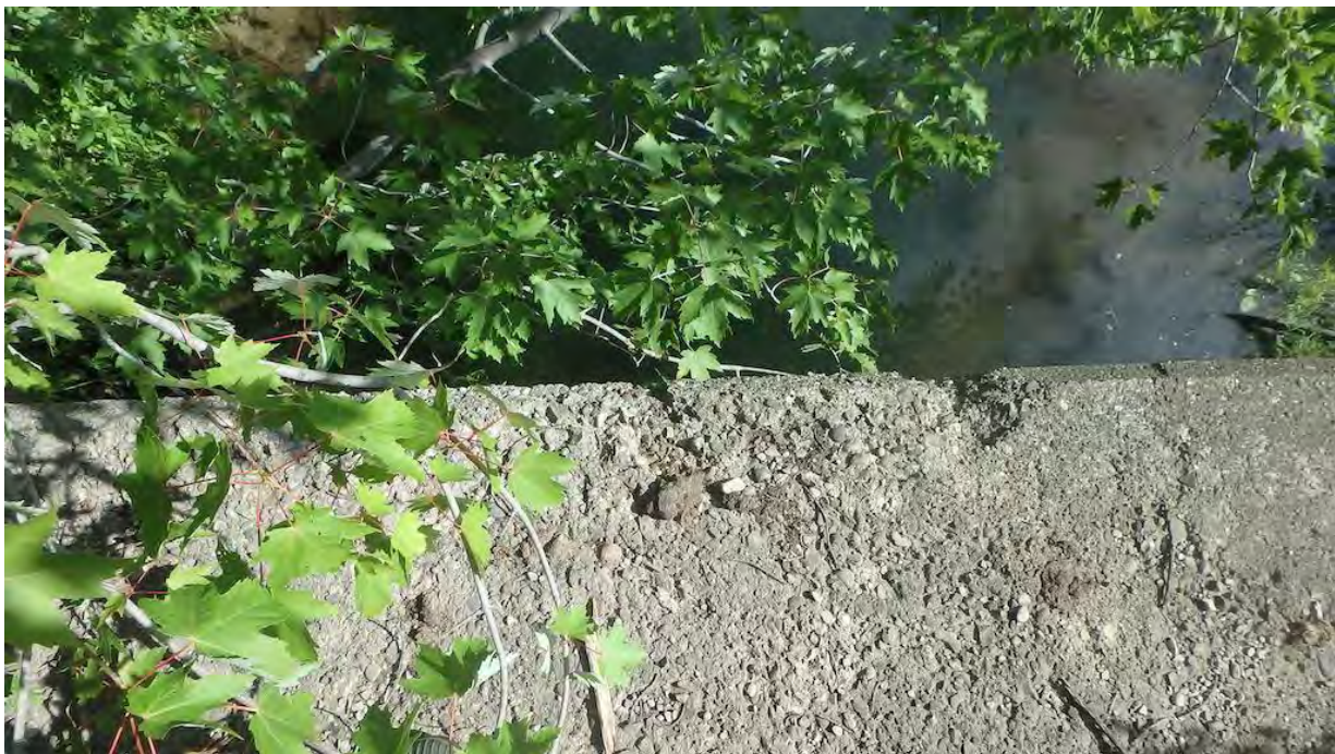
Figure 10 Edge Spalling and Deterioration at Inlet
