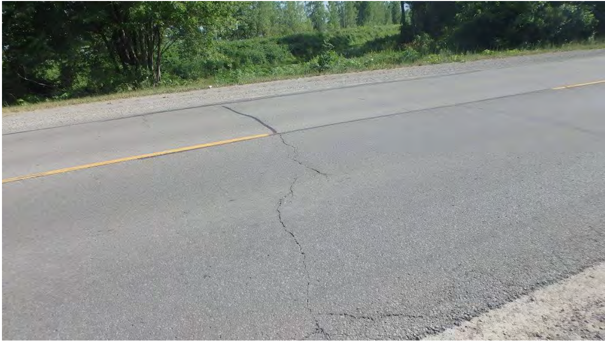
Figure 11 Longitudinal and Transverse Cracks in Wearing Surface
