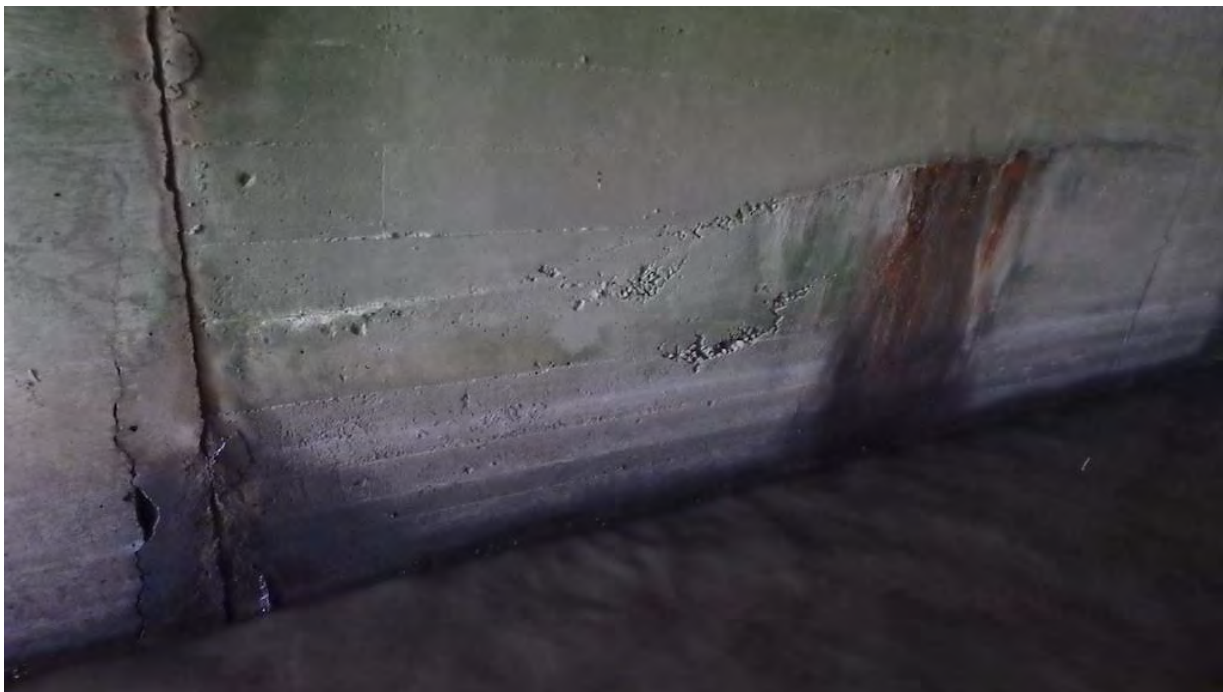
Figure 10 Narrow Crack and Staining at South Wall
