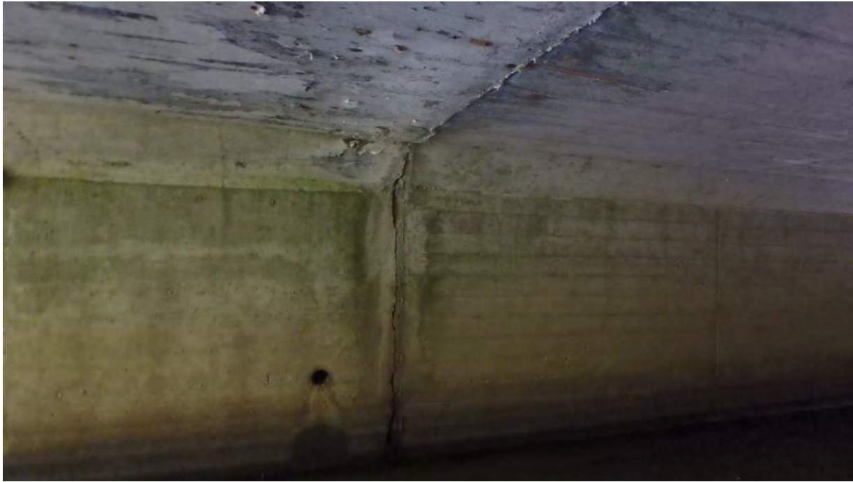
Figure 11 Leakage at Joints
