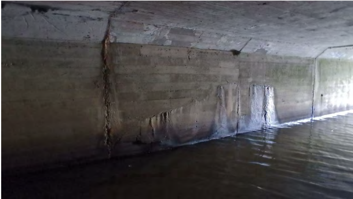
Figure 9 Narrow Crack and Staining at North Wall
