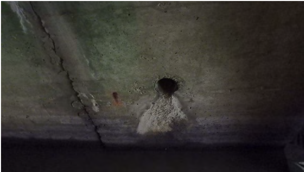
Figure 12 Typical Deterioration at Drains
