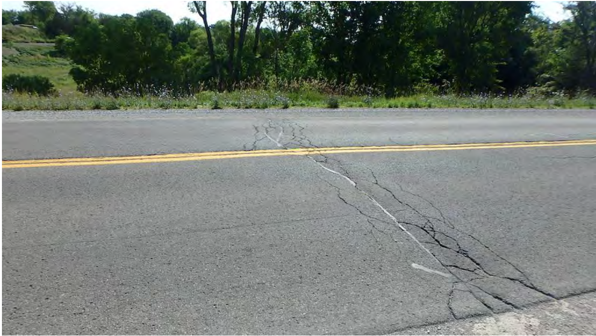
Figure 13 Wearing Surface, Note Transverse Crack
