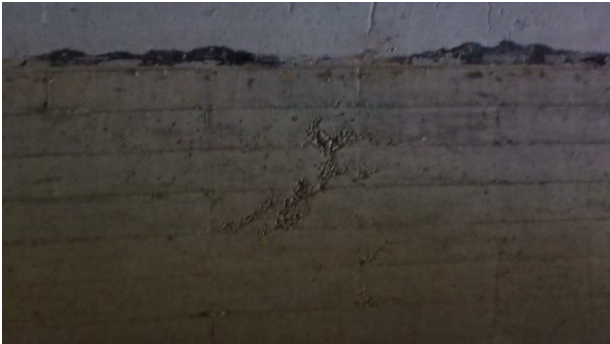
Figure 8 Honeycombing at North Wall
