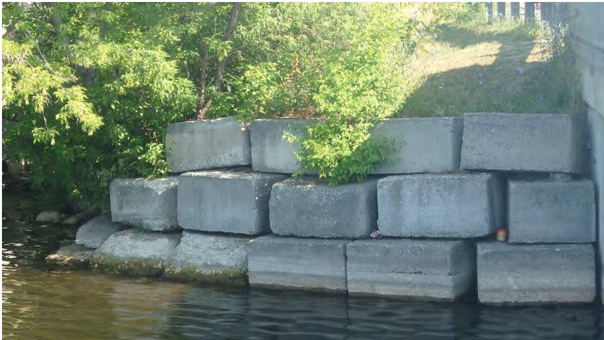
Figure 10 Separation of Retaining Wall
