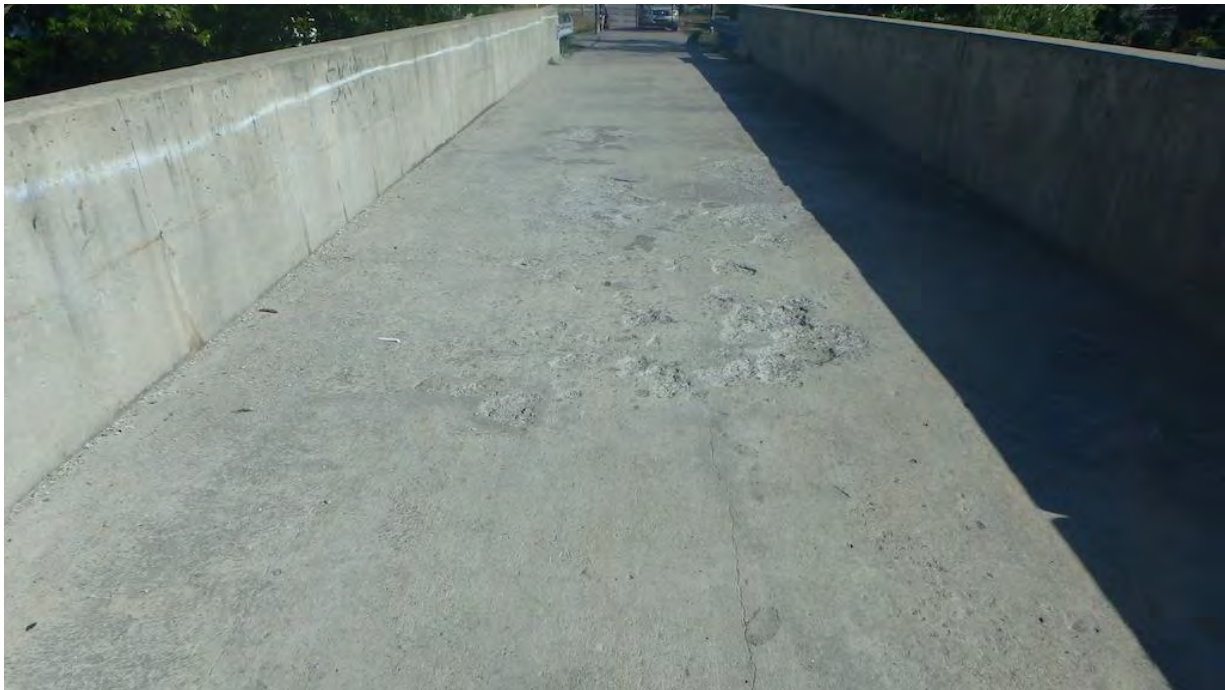
Figure 12 Potholes and Longitudinal Cracks in Deck
