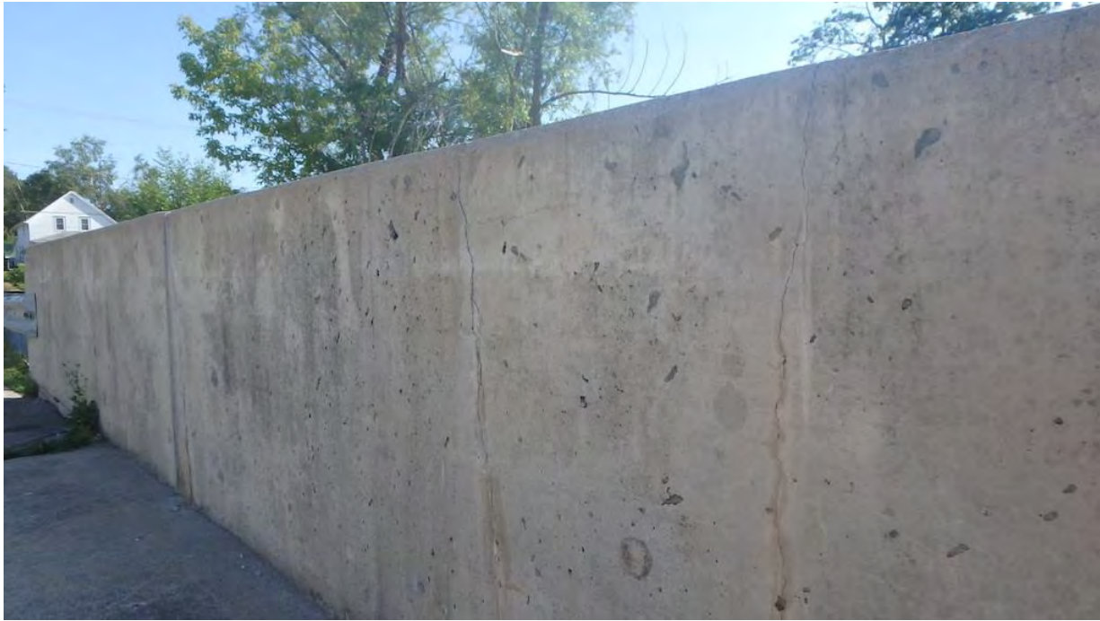
Figure 11 Typical Vertical Cracks in Barrier Walls
