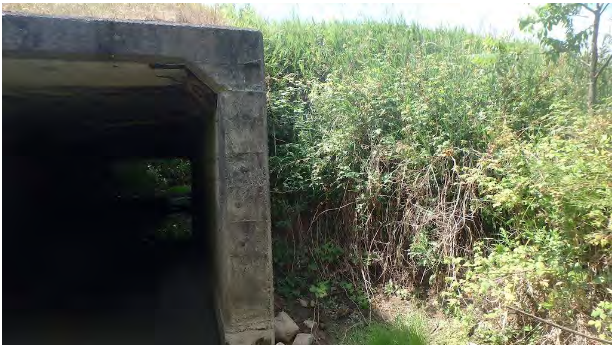
Figure 10 Erosion at Northwest Quadrant
