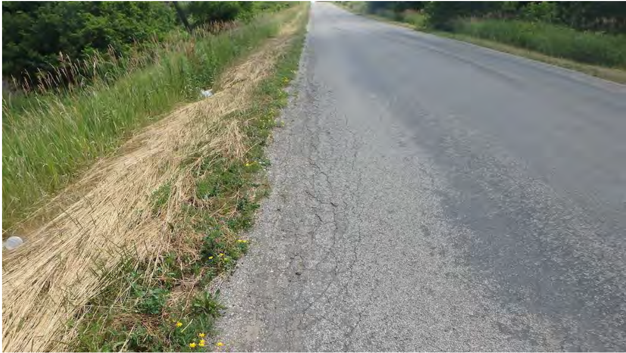
Figure 11 Cracking and Rutting at Edges of Wearing Surface
