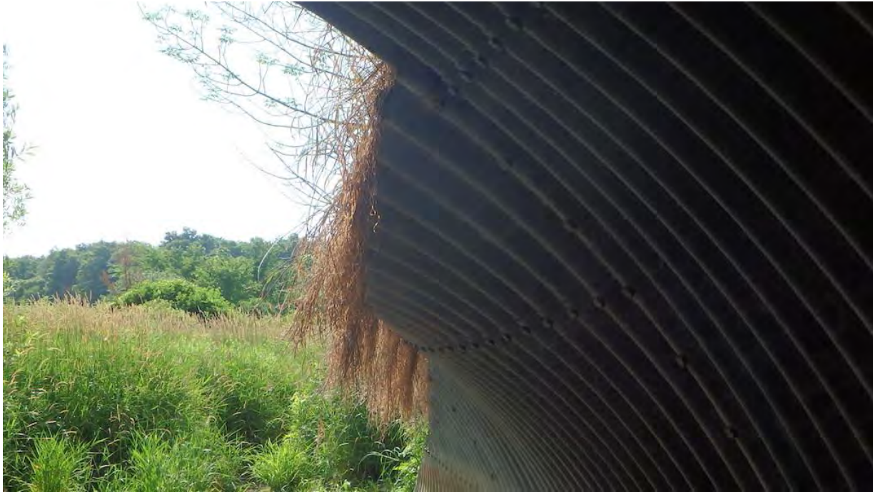
Figure 11 Deflected Culvert Ends at all Quadrants
