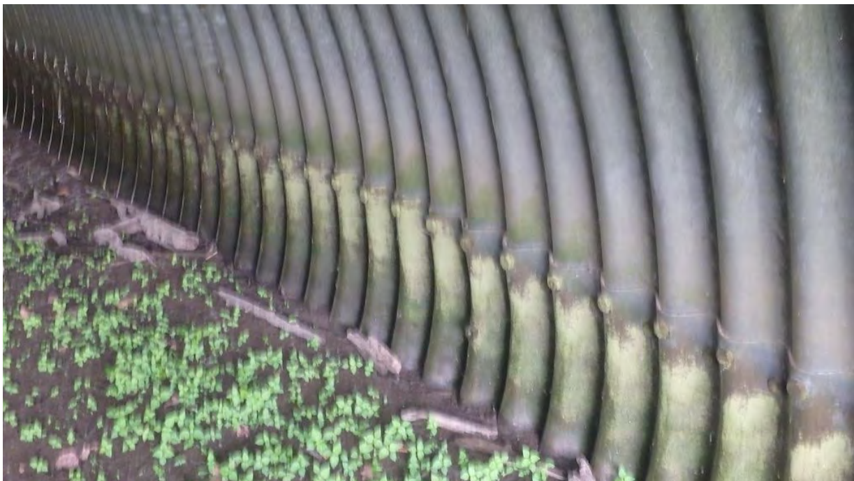
Figure 10 Typical Surface Corrosion in Barrel
