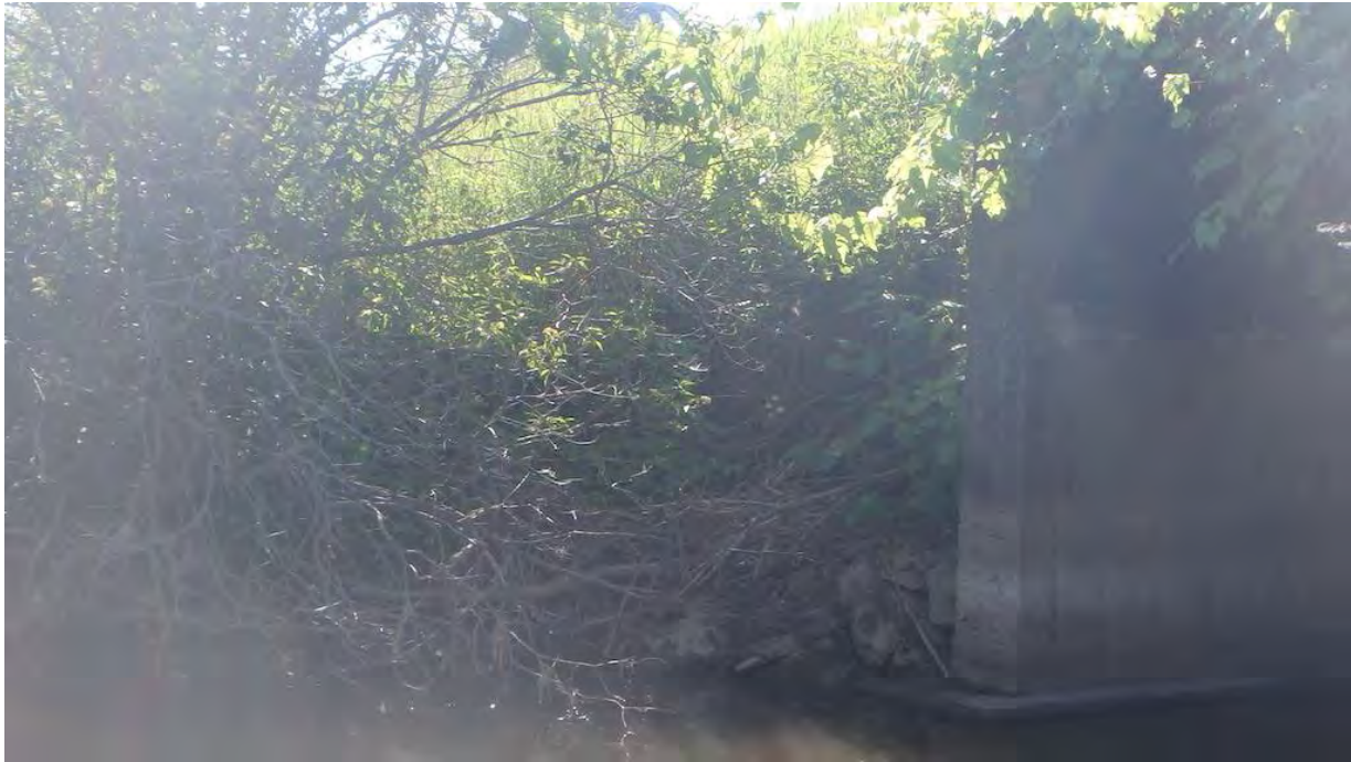
Figure 9 Minor Erosion at Northeast Quadrant
