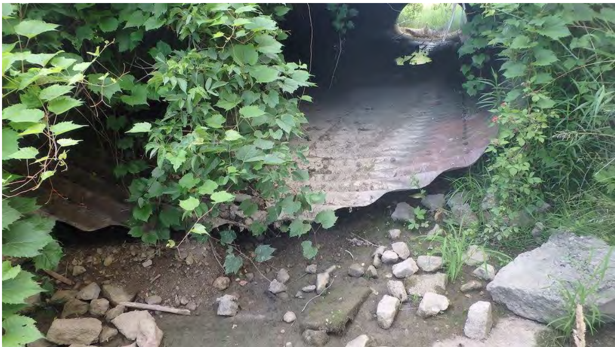
Figure 10 Undermining at Outlet
