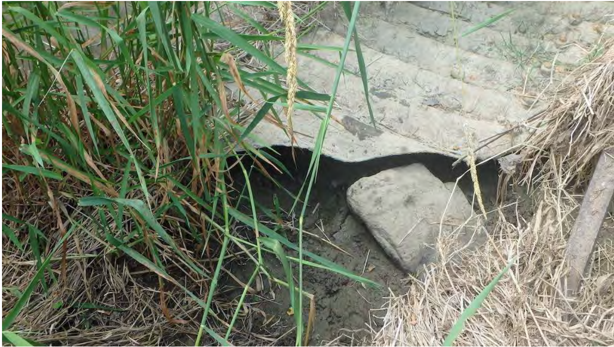
Figure 9 Undermining at Inlet
