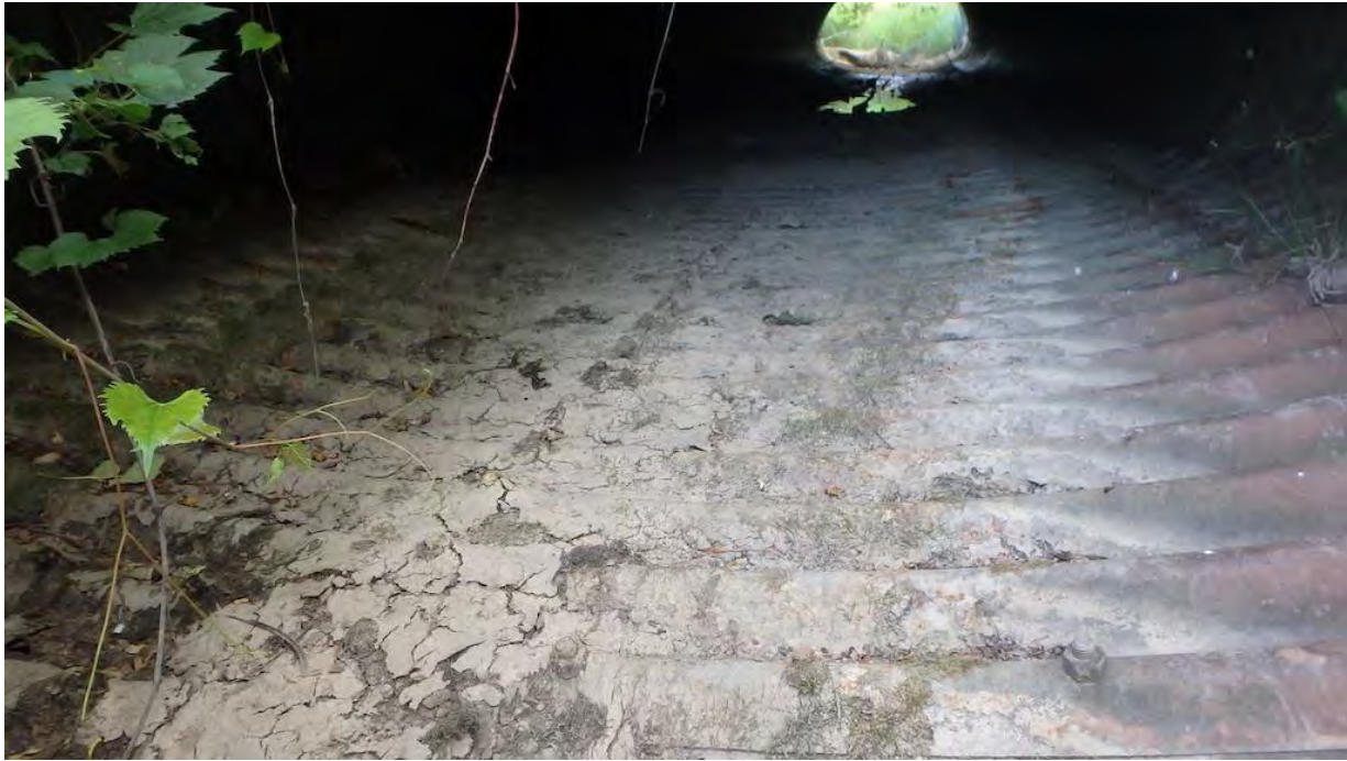
Figure 11 Typical Corrosion on Culvert Bottom
