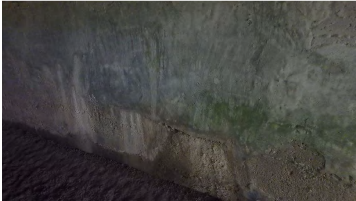
Figure 9 Typical Scaling and Leakage on Culvert Walls
