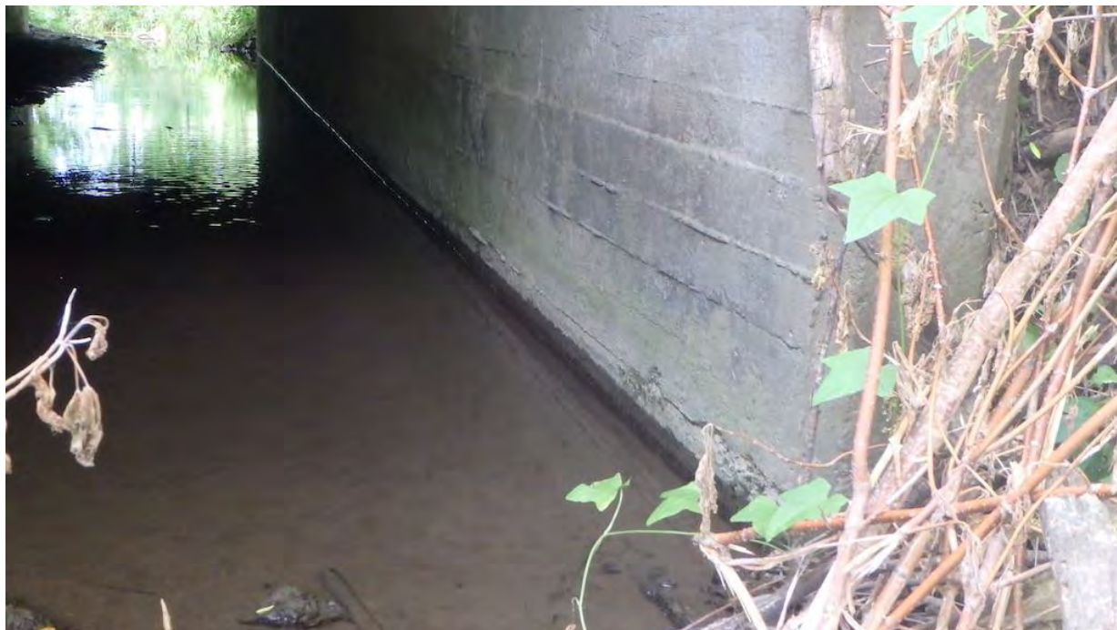
Figure 10 Typical Scaling and Spalling on Culvert Walls
