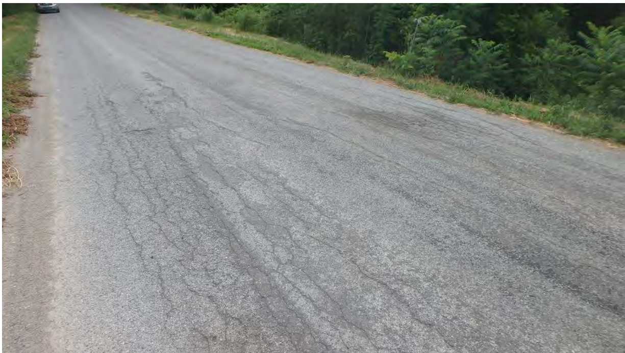
Figure 10 Alligator Cracking and Rutting at Edges of Wearing Surface
