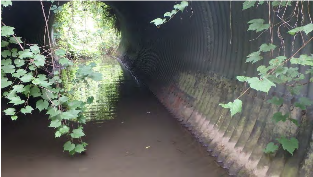
Figure 9 Surface Corrosion in Barrel
