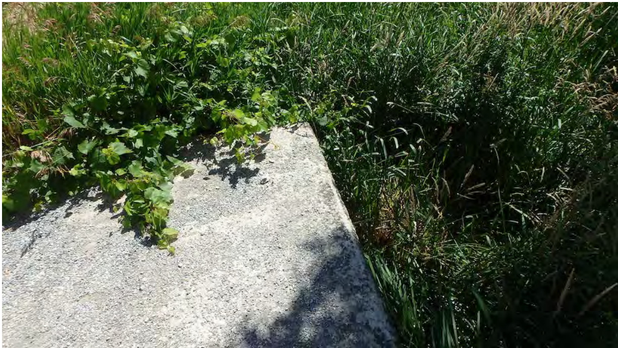
Figure 10 Moderate Spalling on Top of Culvert
