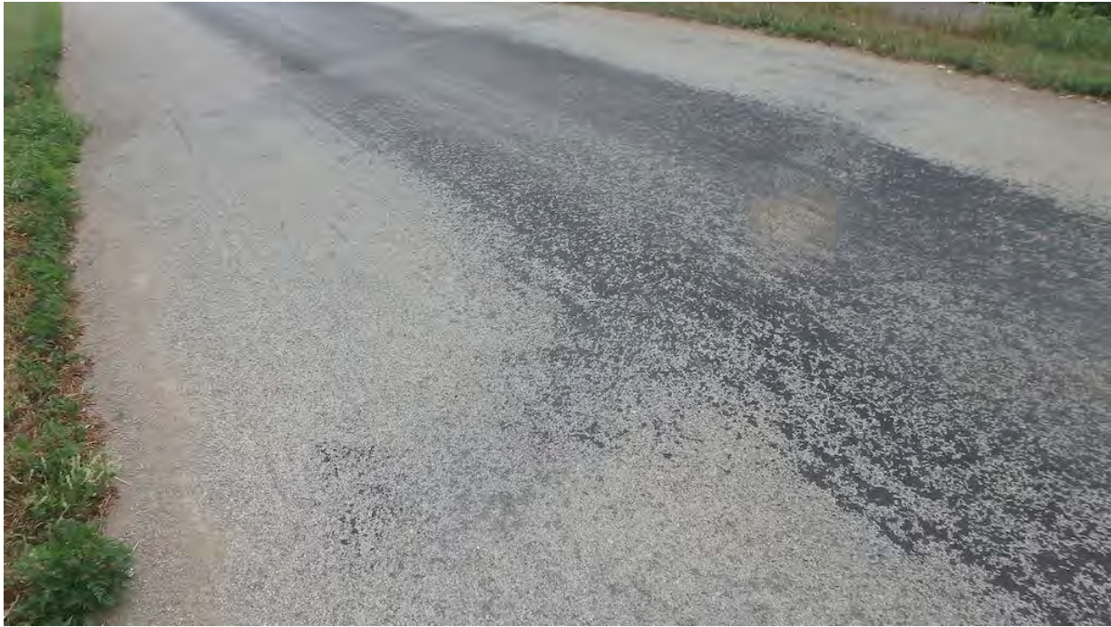
Figure 11 Polishing and Settlement of Wearing Surface at Culvert
