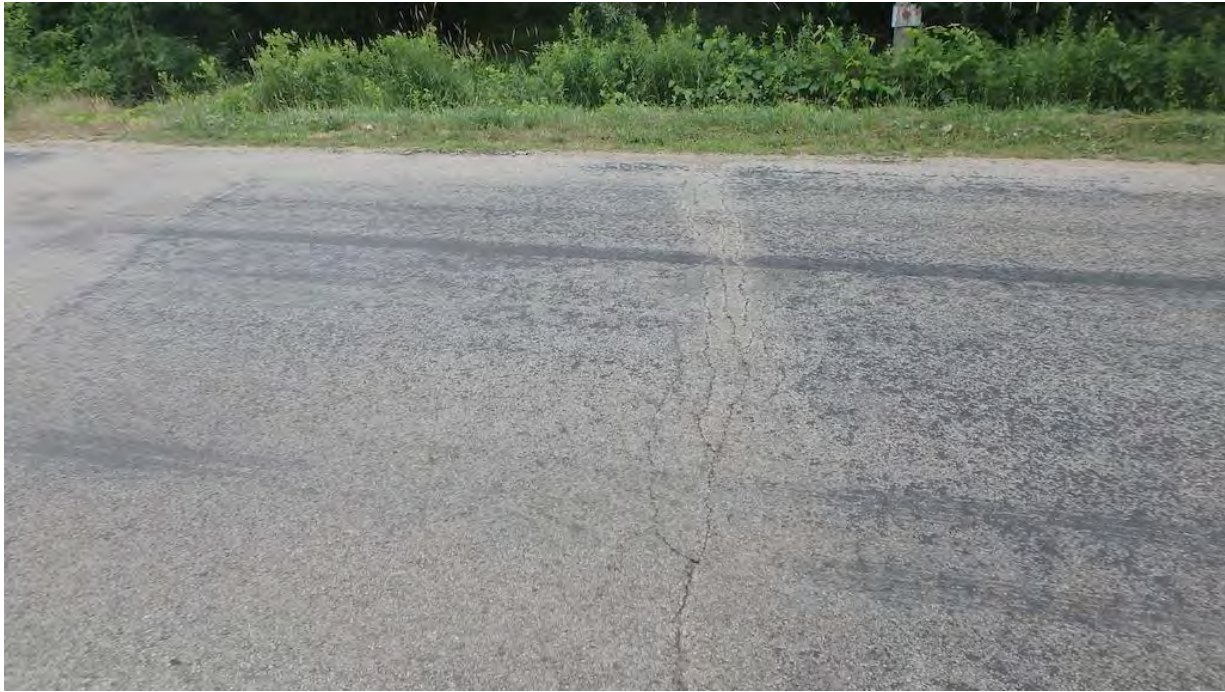
Figure 9 Longitudinal and Transverse Cracking in Wearing Surface
