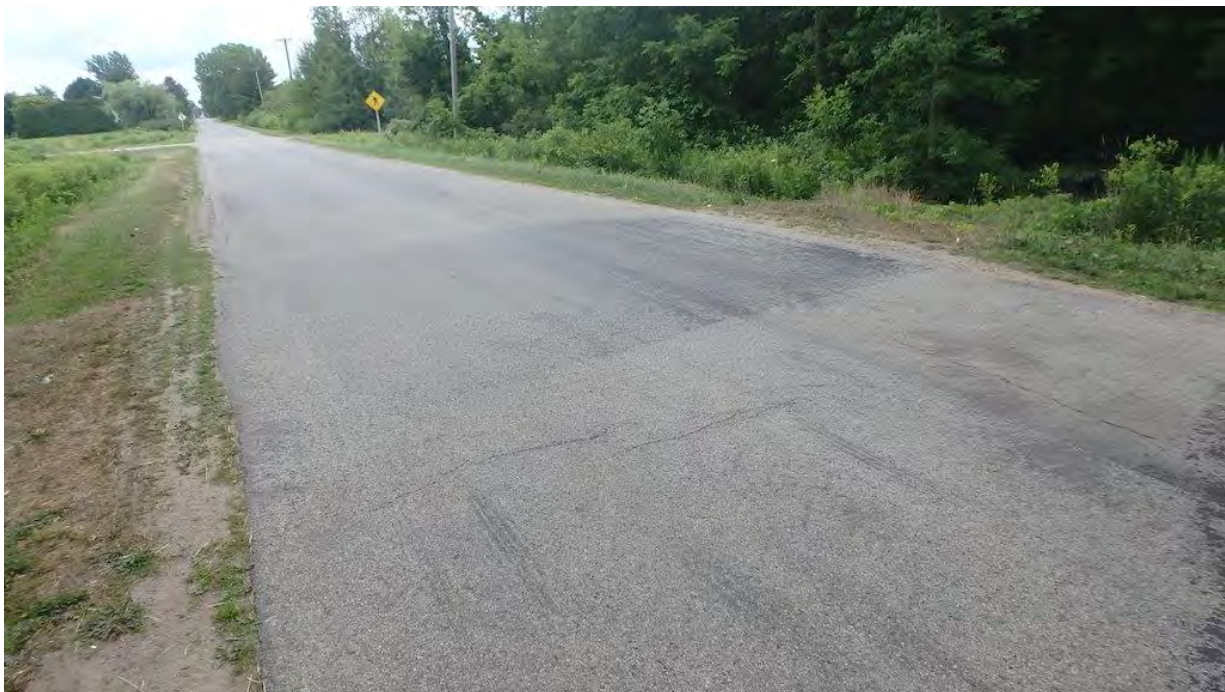
Figure 8 Settlement in Wearing Surface at Culvert
