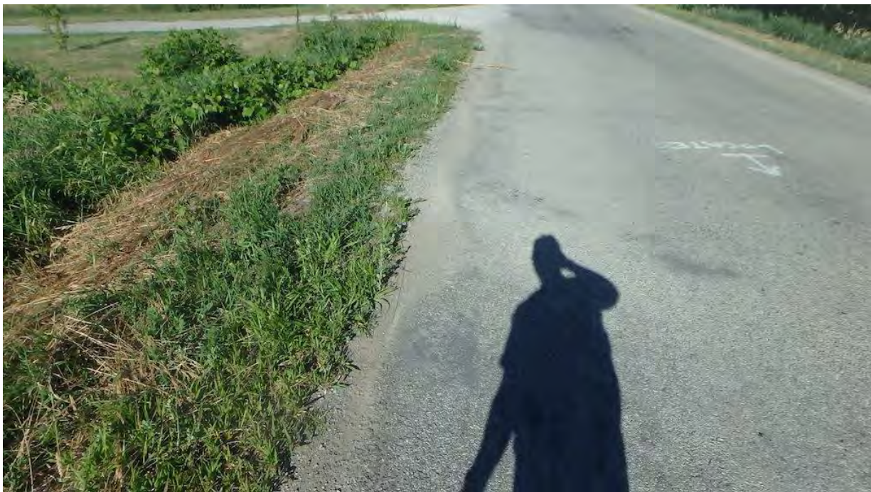
Figure 10 Minor Erosion of Asphalt Wearing Surface
