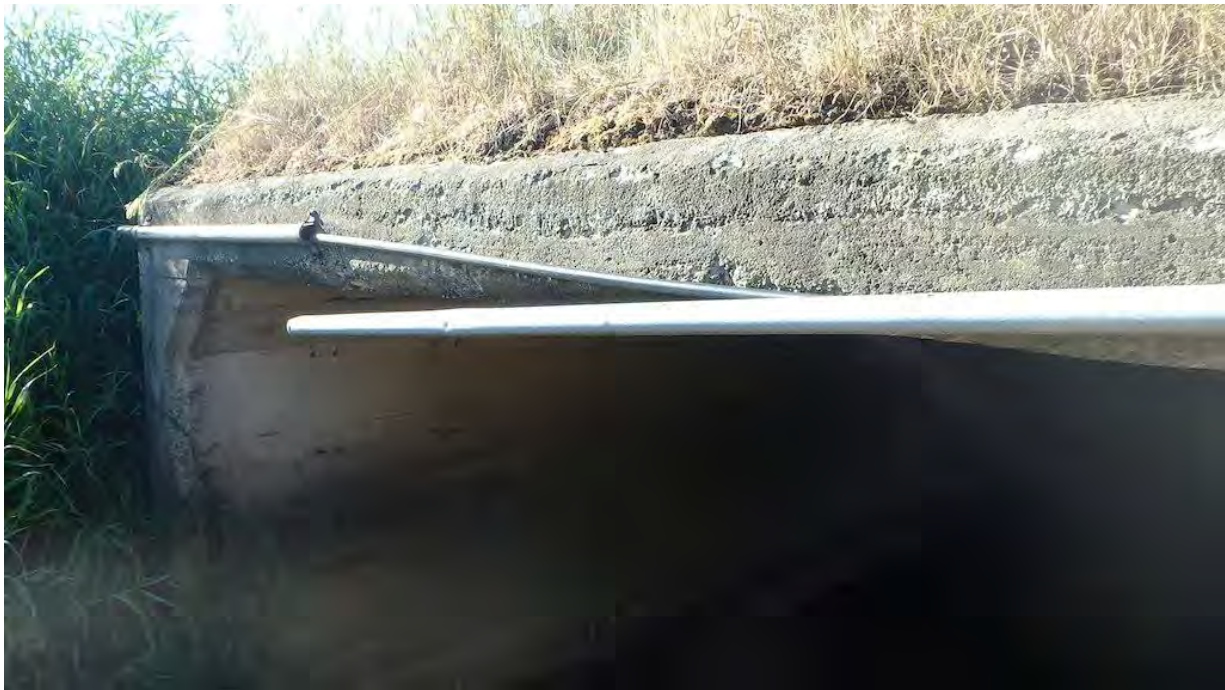
Figure 8 Detached Conduit on North Fascia
