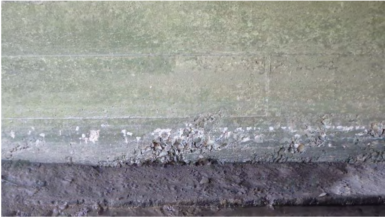
Figure 9 Minor Scaling and Honeycombing on East Wall
