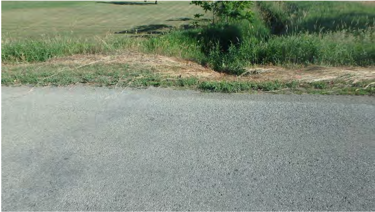
Figure 11 Minor Settlement of Wearing Surface at Structure Edges
