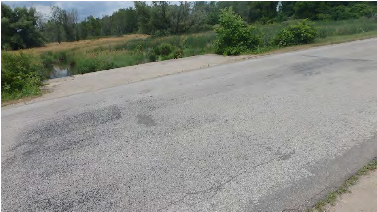
Figure 9 Settlement in Wearing Surface at Culvert
