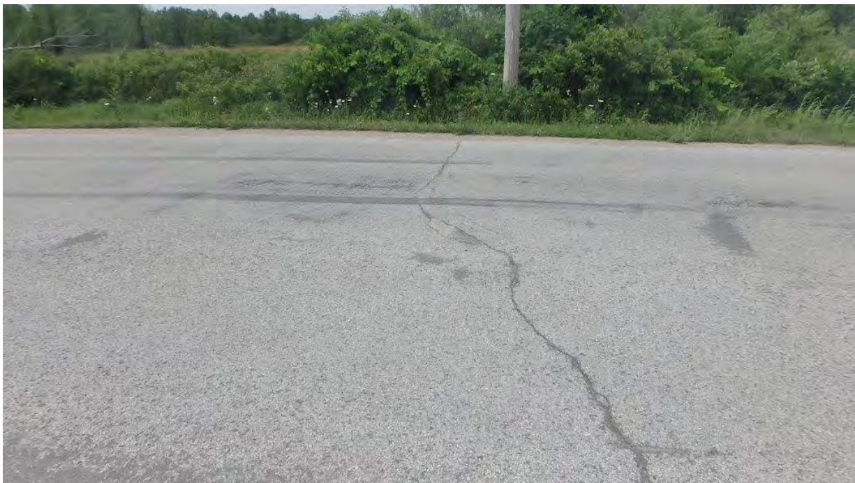
Figure 10 Transverse Crack at West Approach
