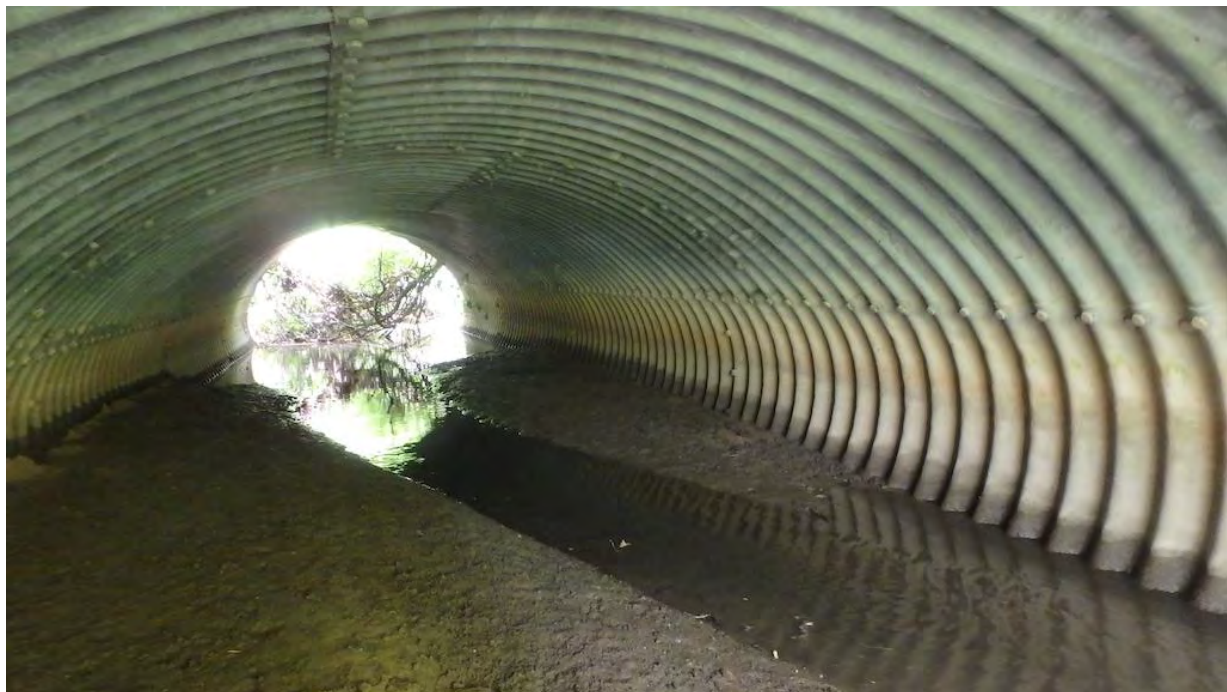
Figure 8 Minor Surface Corrosion
