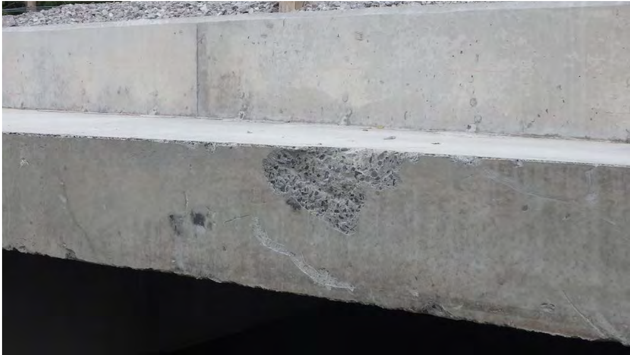
Figure 9 Light Impact Damage on North Fascia
