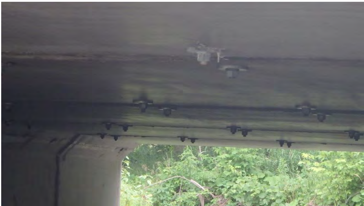
Figure 10 Light Leakage with Chlorides at Bolts in Soffit
