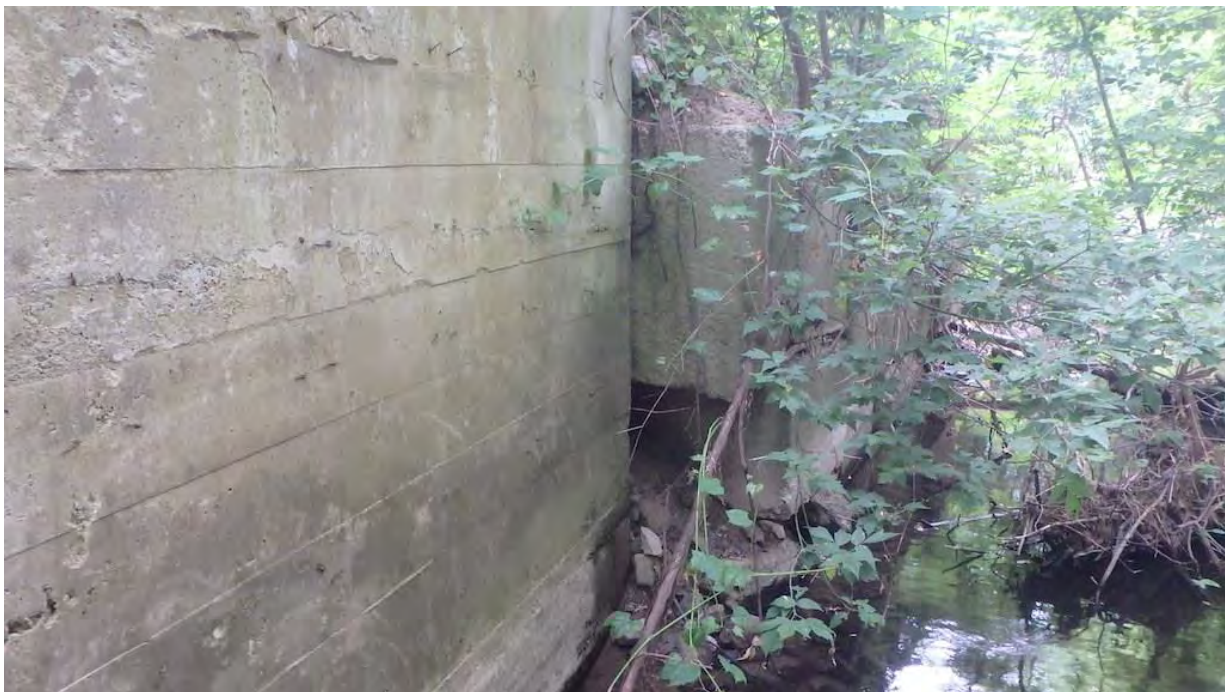
Figure 12 Minor Erosion at Northwest Quadrant
