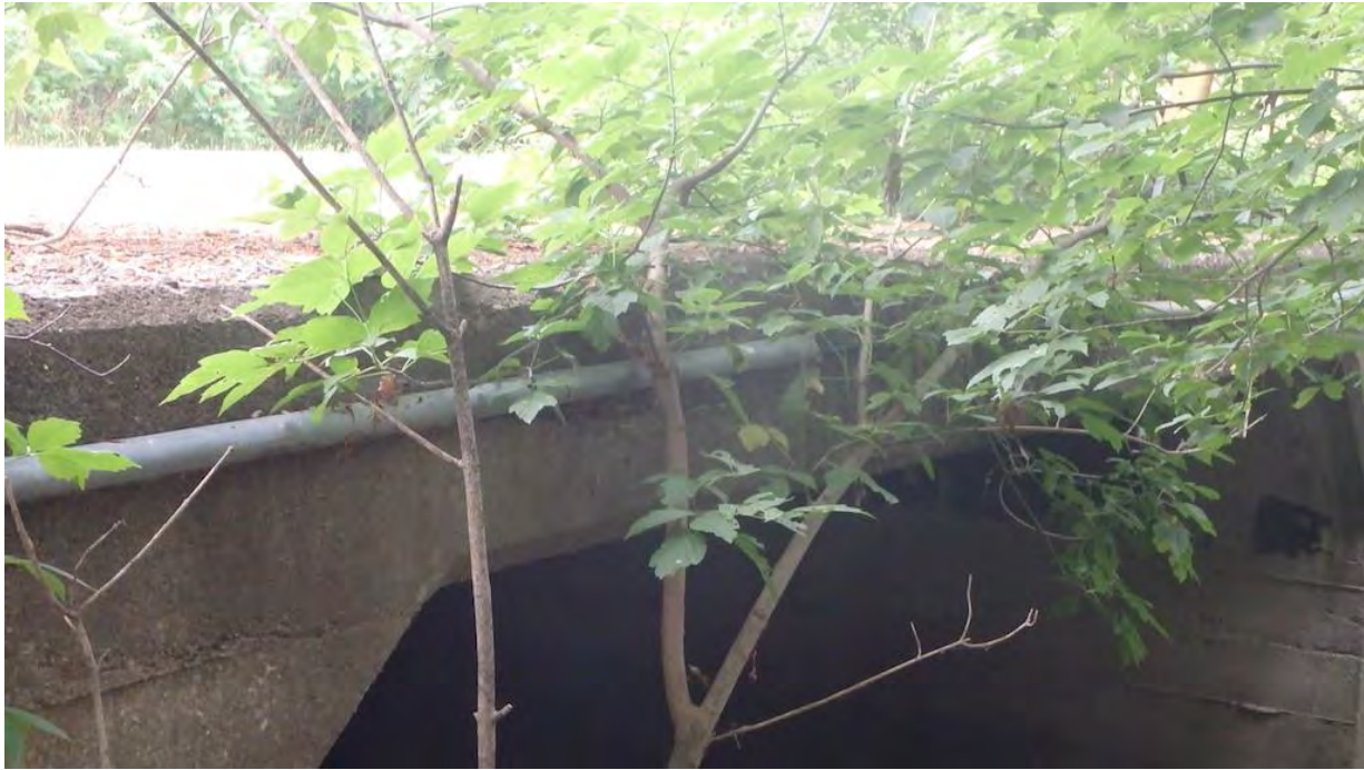
Figure 11 Damaged Utility Cable on South Fascia
