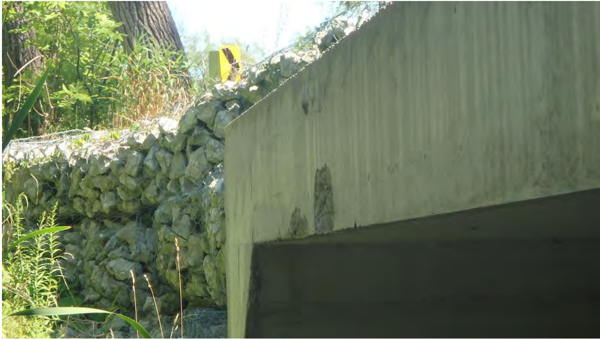
Figure 9 Small Impact Damage on East Fascia
