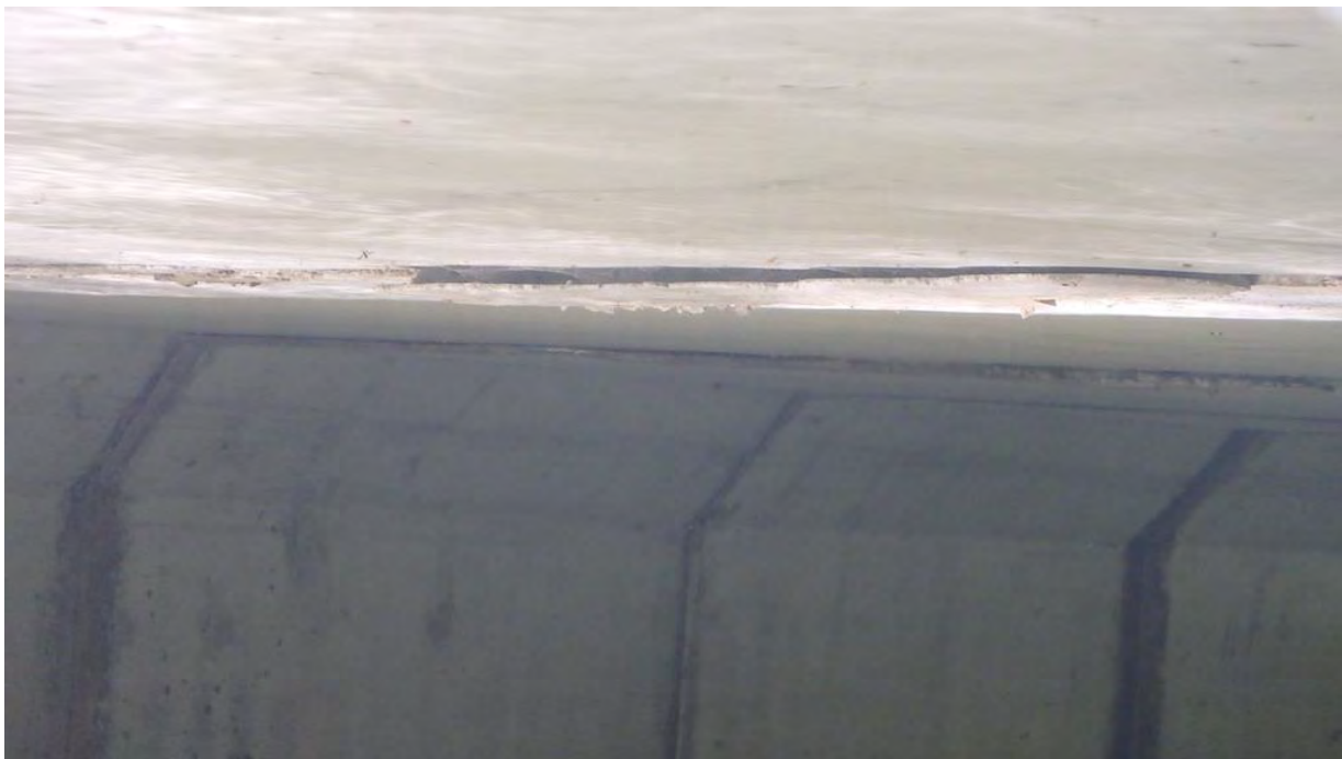
Figure 10 Deterioration of Parging at Joints
