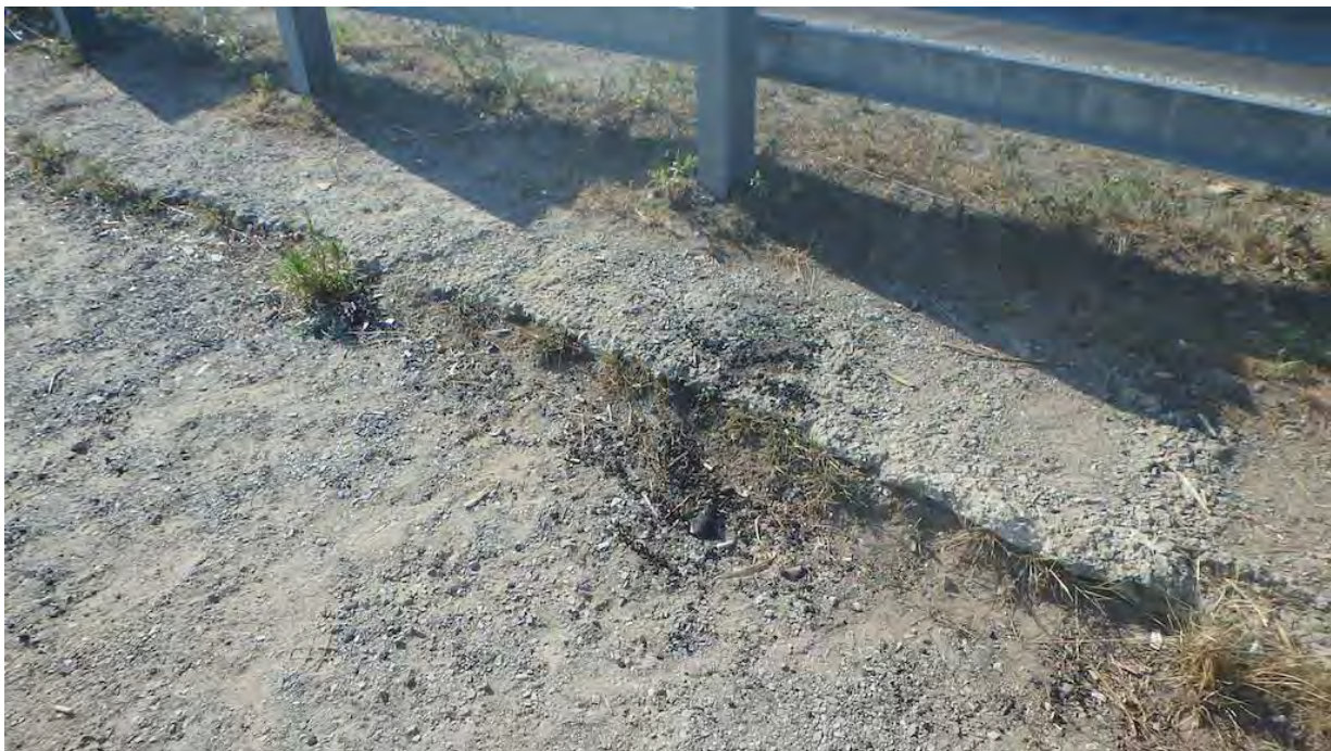
Figure 8 Typical Spalling at Outside Curb Edges
