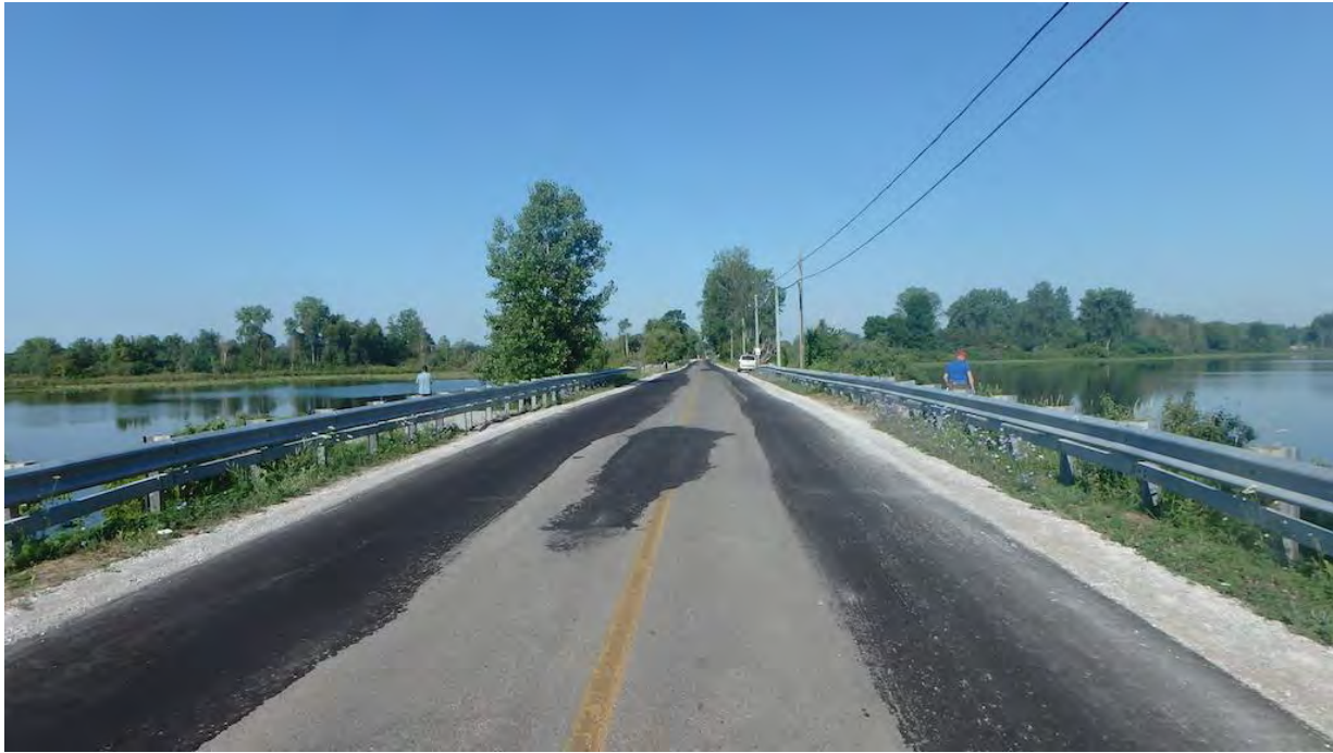
Figure 7 Patching and Centreline Crack in Wearing Surface
