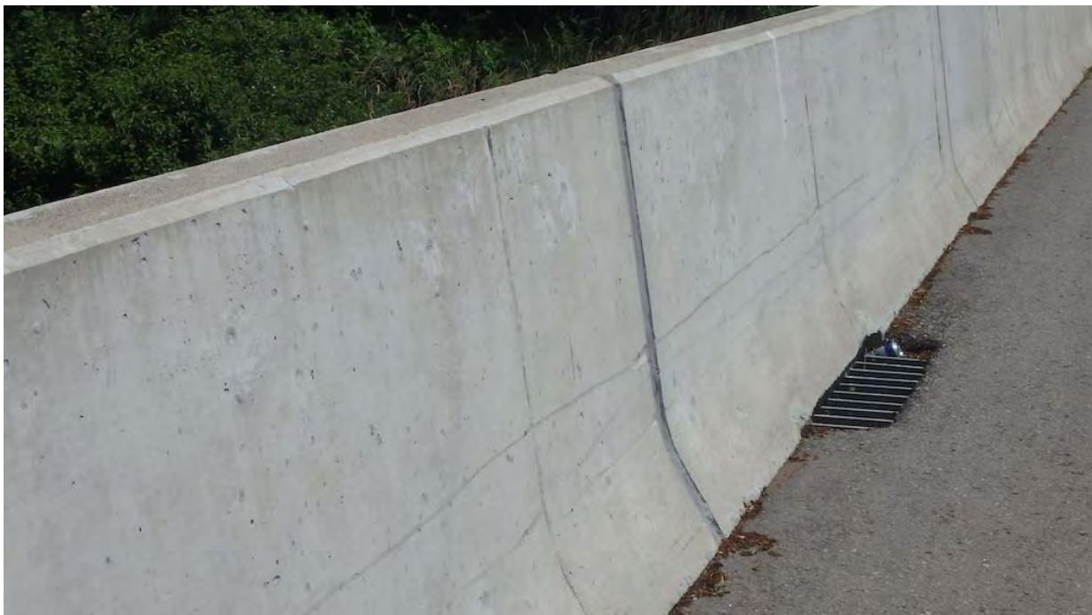
Figure 10 Slight Impact Damage on Barriers
