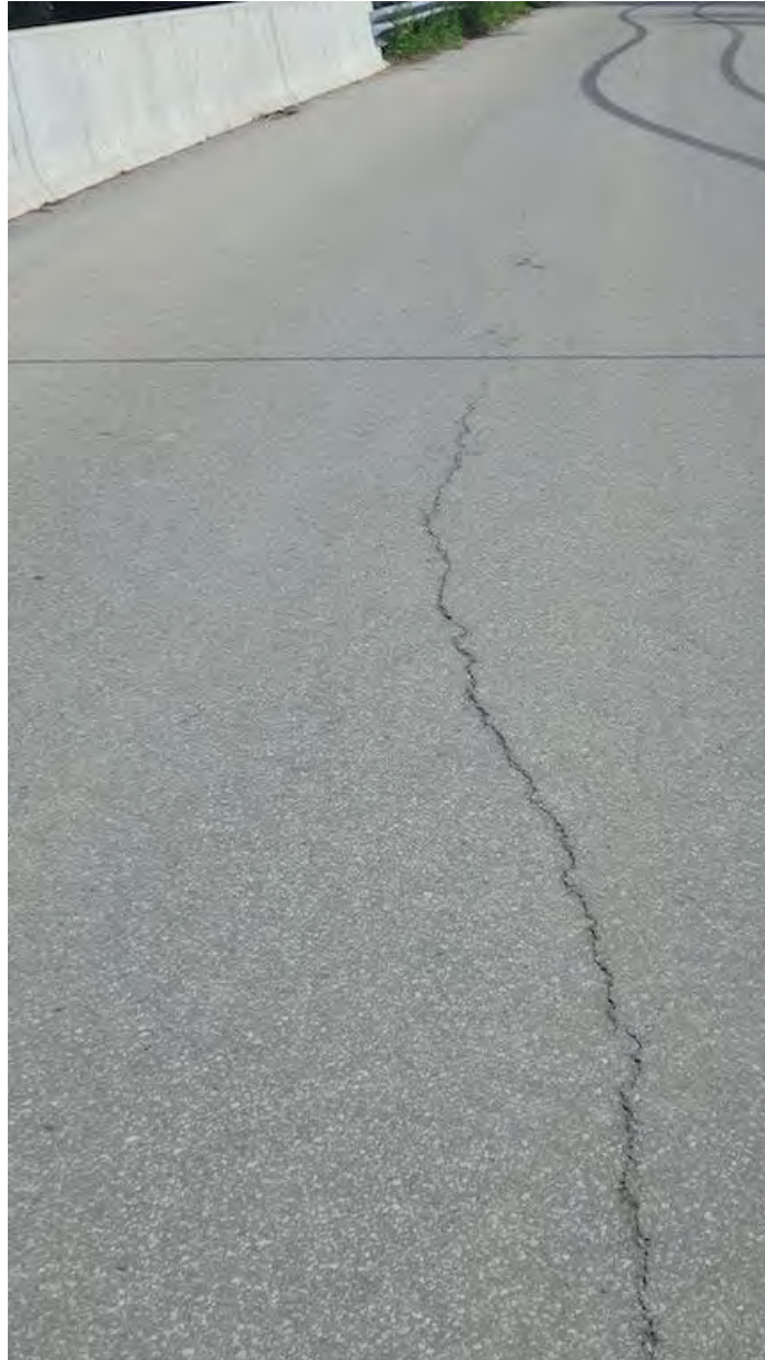
Figure 11 Longitudinal Crack in Wearing Surface
