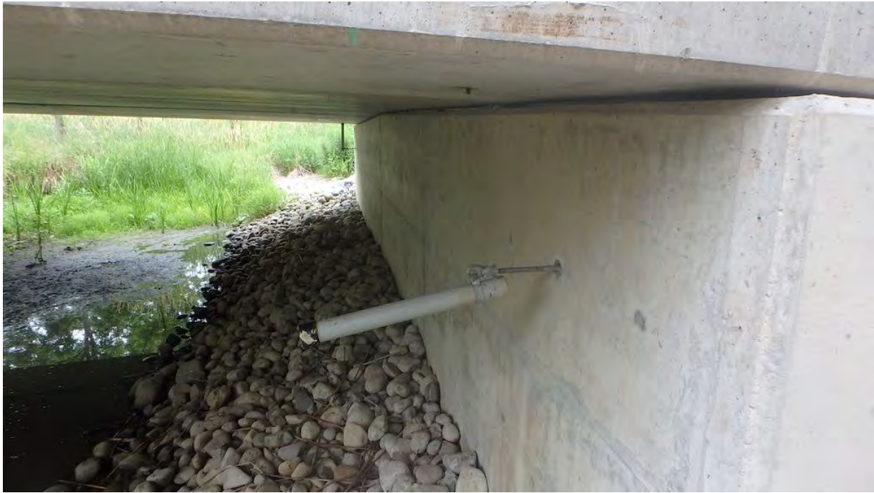
Figure 12 Broken Asphalt Drain at Southeast Quadrant
