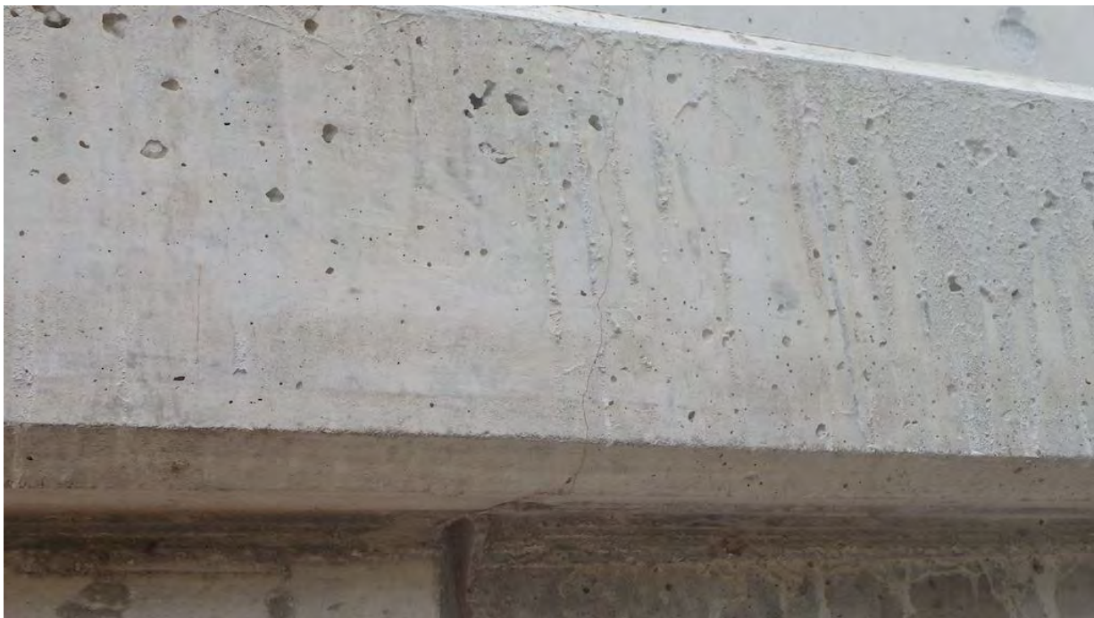
Figure 10 Typical Hairline Crack in Fascia
