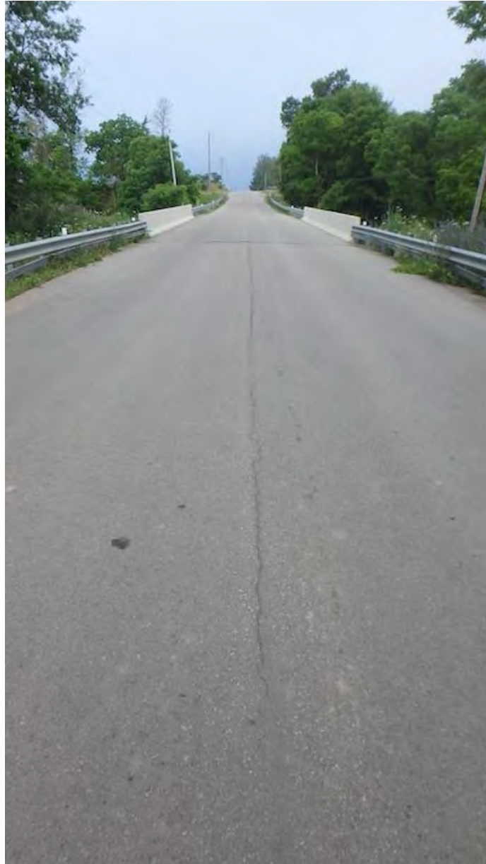
Figure 11 Centreline Longitudinal Crack in Wearing Surface
