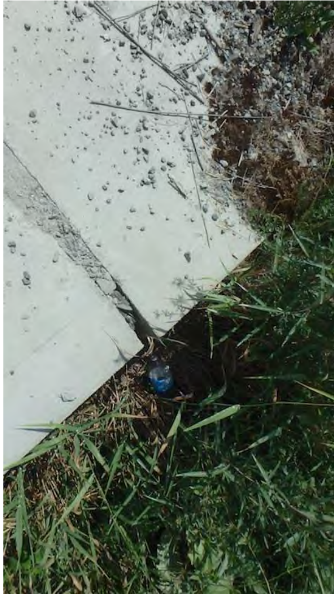
Figure 9 Minor Loss of Parging at Northwest Quadrant
