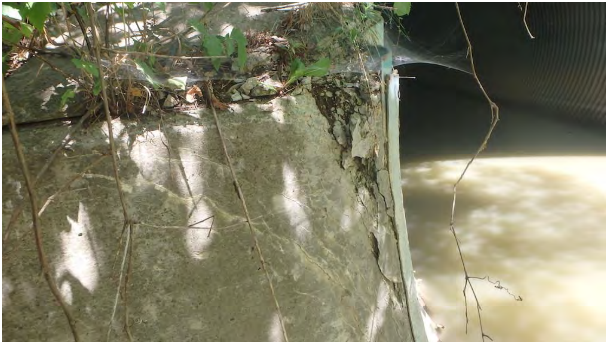
Figure 10 Delamination and Spalling at Southwest Quadrant
